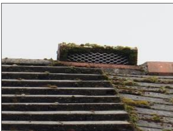
exploitable gaps under the flashing.
