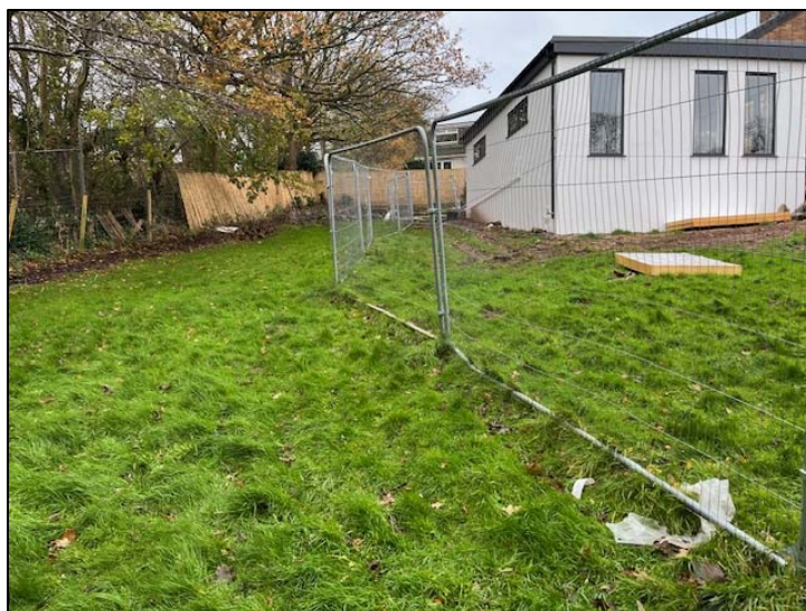
Figure 1: This image shows the new extension and it is clear that no construction works have taken place beyond the tree protection fencing.
