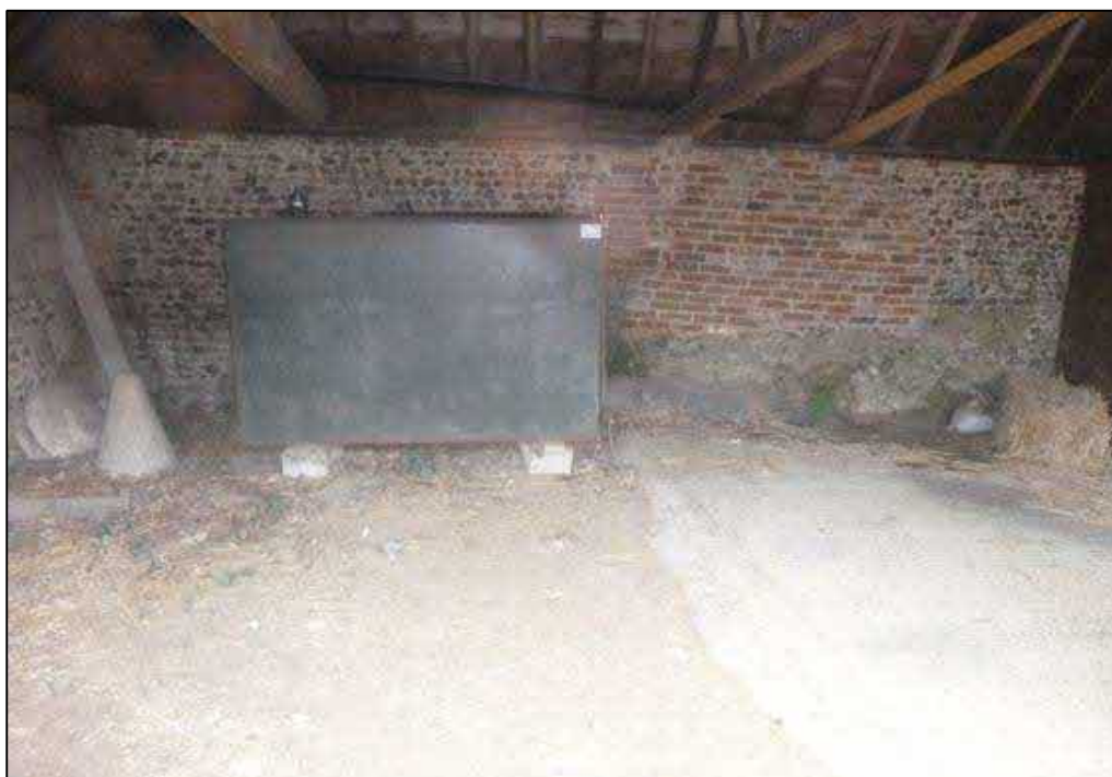
Photograph 3 Showing the oil tank within Building A
