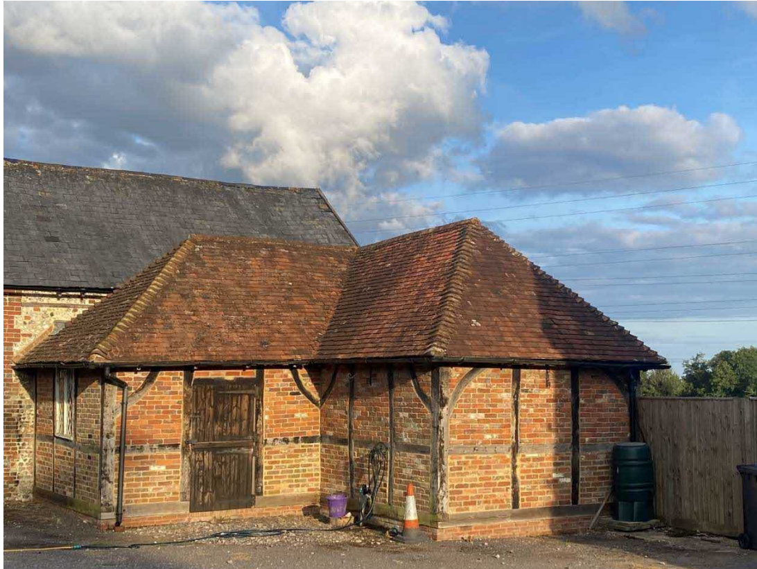
Figure 12. Northern and western elevations of south building looking east. extension looking south. All faces of the roof have numerous potential access point for bats.
