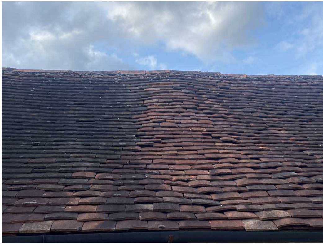
Figure 9. Detail of northern face of Middle building showing numerous potential access point for bats.
