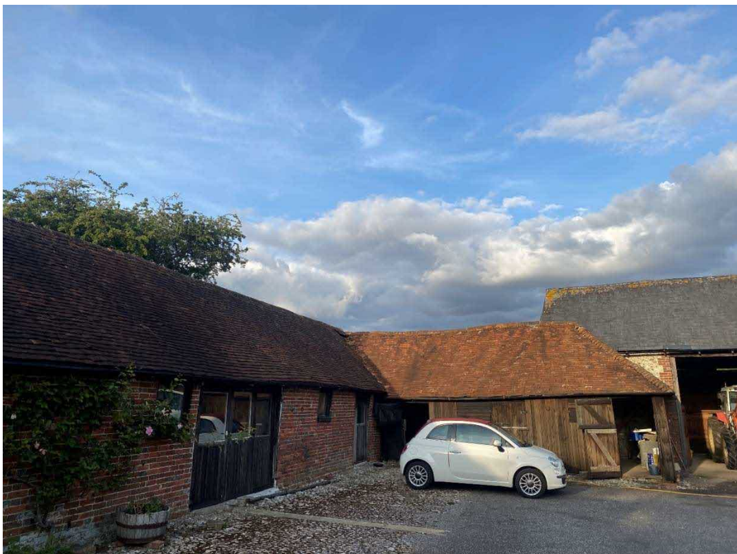
Figure 6. Middle Building Western and southern elevations (eastern two-thirds) looking northeast. Red arrow indicates potential access point for bats.
