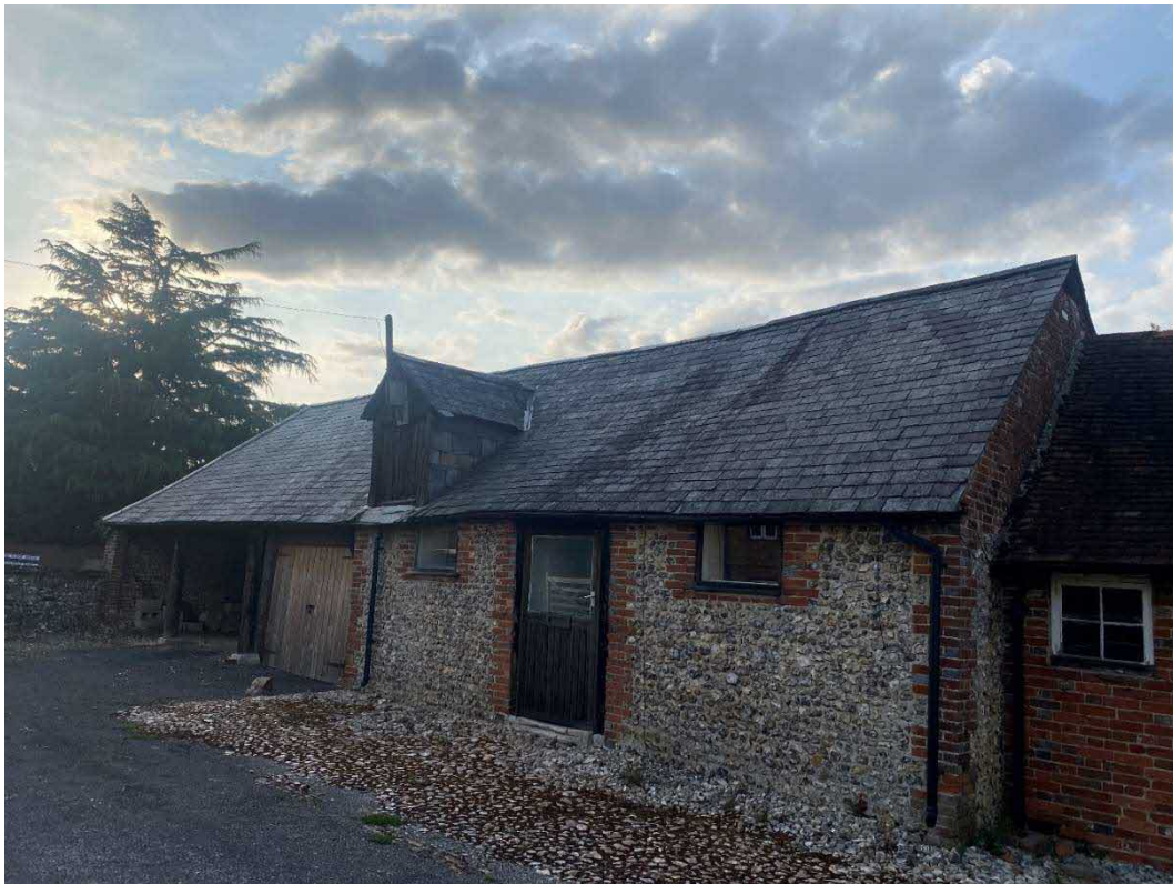
Figure 2. Western and southern elevations of West Barn looking northwest. Red arrow indicates potential access point for bats.
