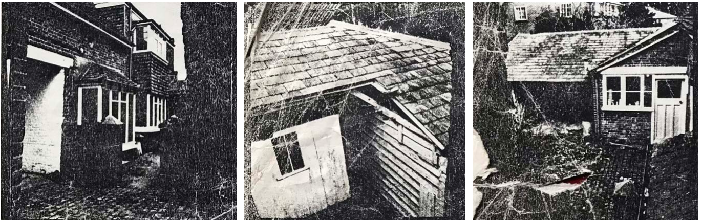
1975 Photos of the site in poor condition
