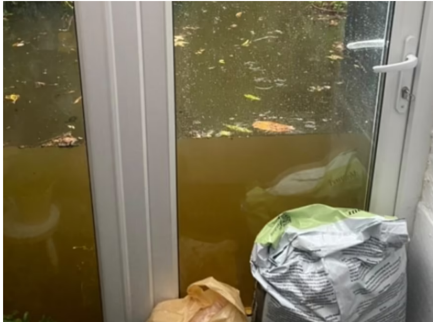
Figure 6: UPVC doors under flood conditions. These appear to offer reasonable flood resilience
