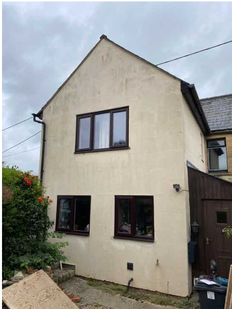
Figure 5 – Weathered render upon existing south elevation
