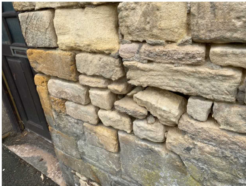
Figure 4 - Damage to north elevation stonework
