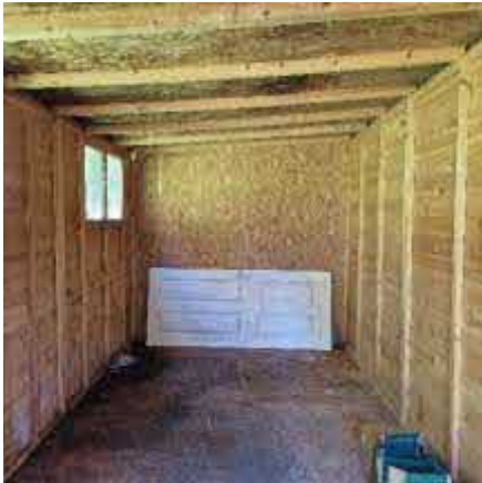
Photograph 3: Internal view of storage areas at the rear of the stable block.
