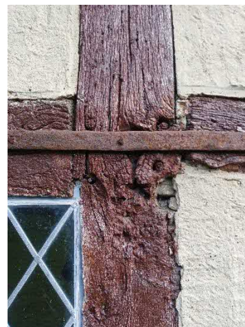
Fig 26. View of poor condition timber and cement lime render.
