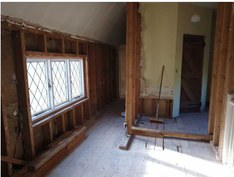
Fig 14. View within adjoining section of later extension looking towards rear wall of 17 th century building.
