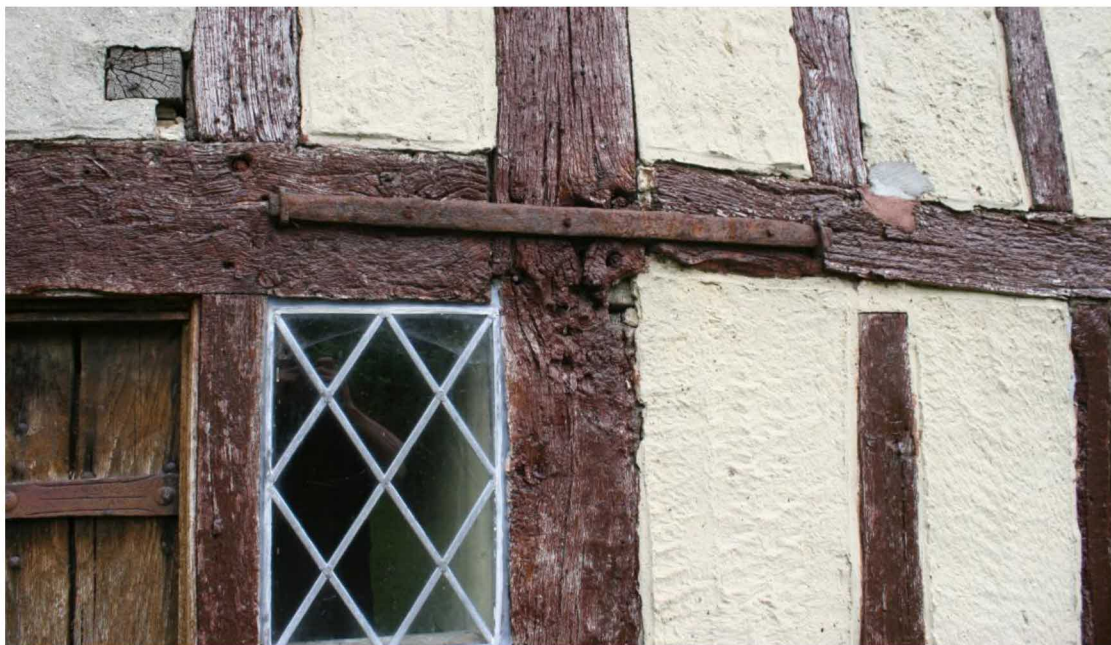
Failing storey post with LC18th or EC19th iron strap repair.
