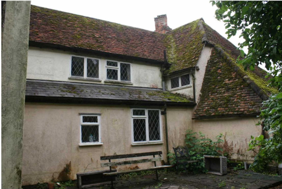
The western elevation of the 1964 extension containing the hall and utility rooms.
