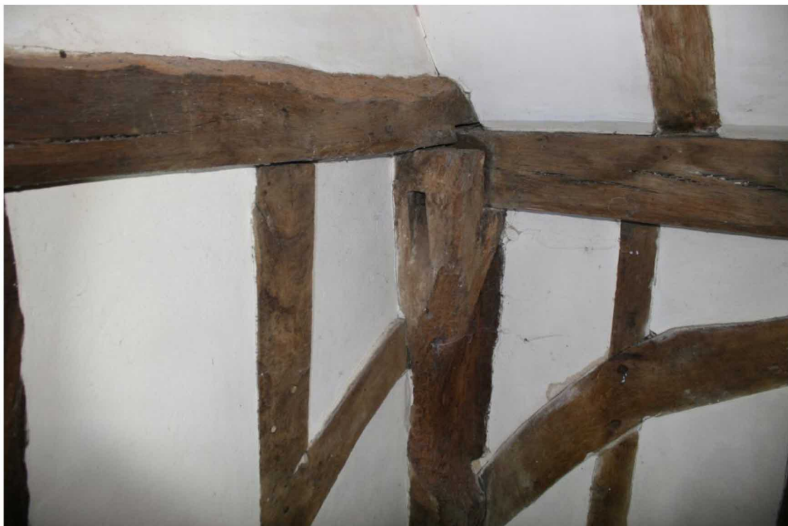
Framing in the SE corner. The corner post has been shaved back.
