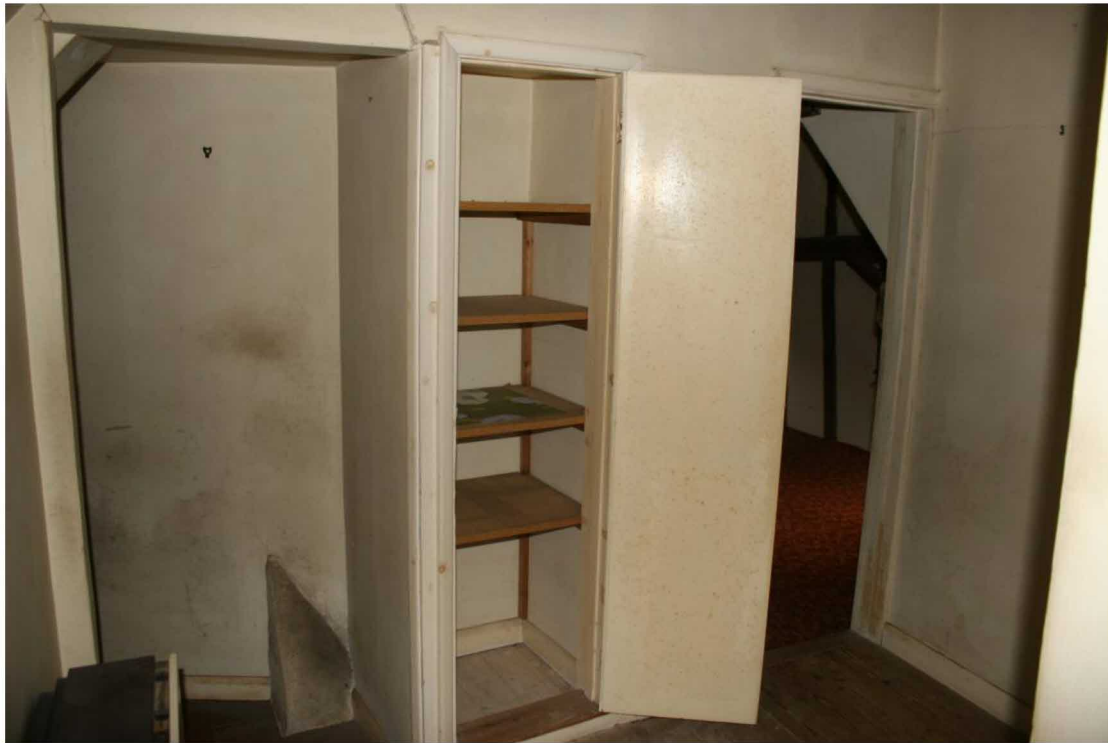
Built in closet beside the firestack on the Landing. Looking S.
