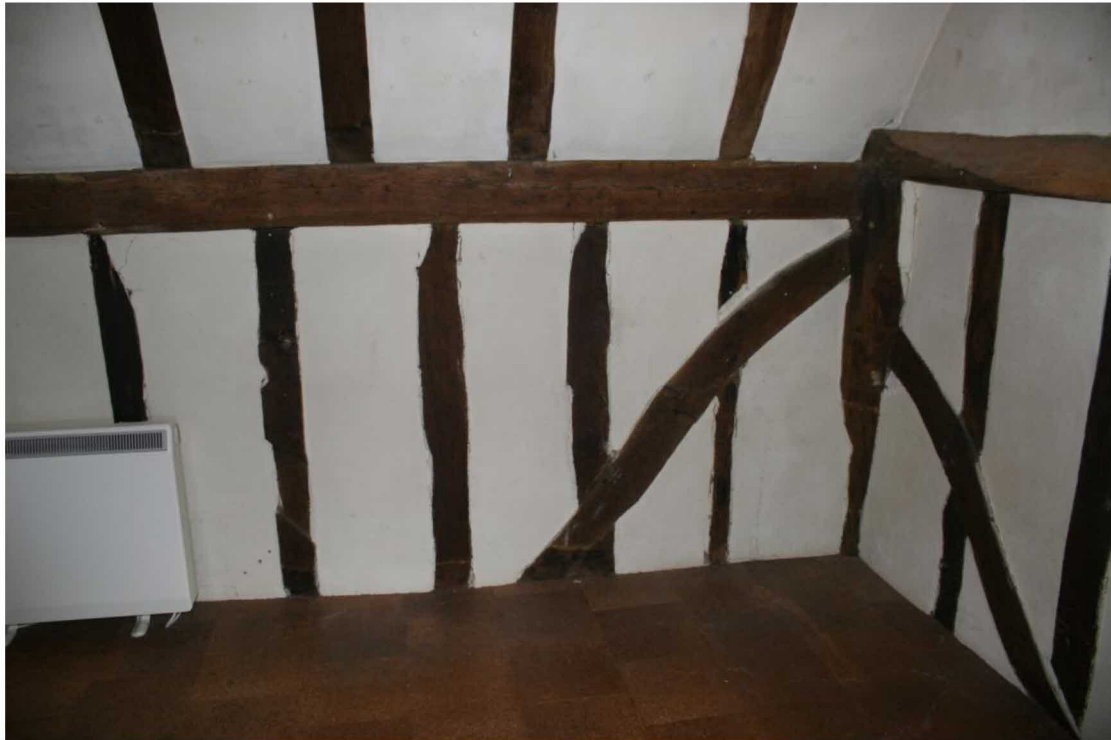
Framing in the NE corner. Note the empty trench for a missing brace.
