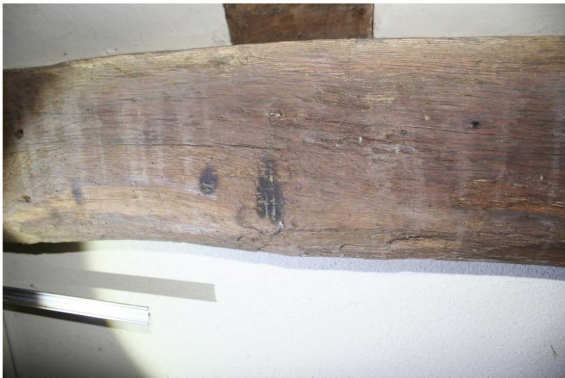
Taper burn marks on the north wall top-plate over the window.
