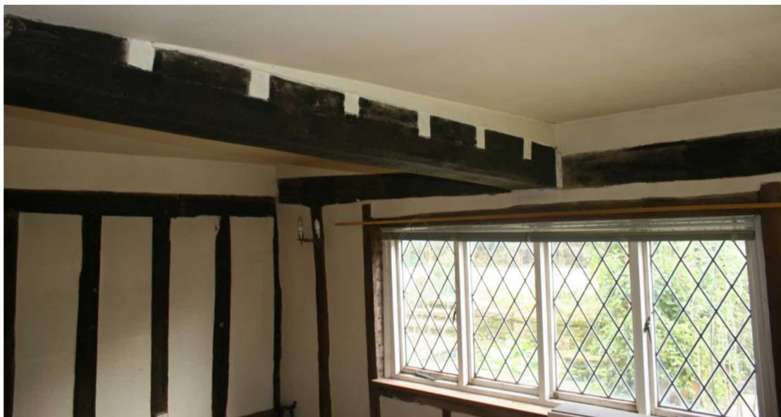
The main joist has sunk and the floor above remade to be level.
