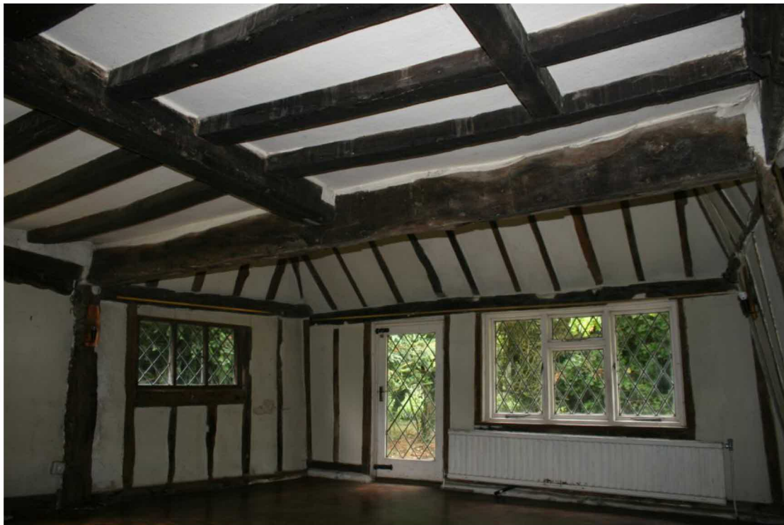
Looking W at the original frame. The end wall has been removed.
