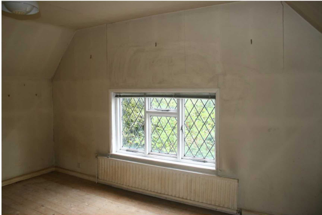
Looking NE in the NE Bedroom. Note the studwork visible in the walls.
