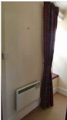
Existing Electric Radiator
