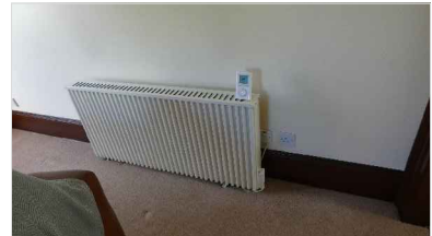
Existing Electric Radiator
