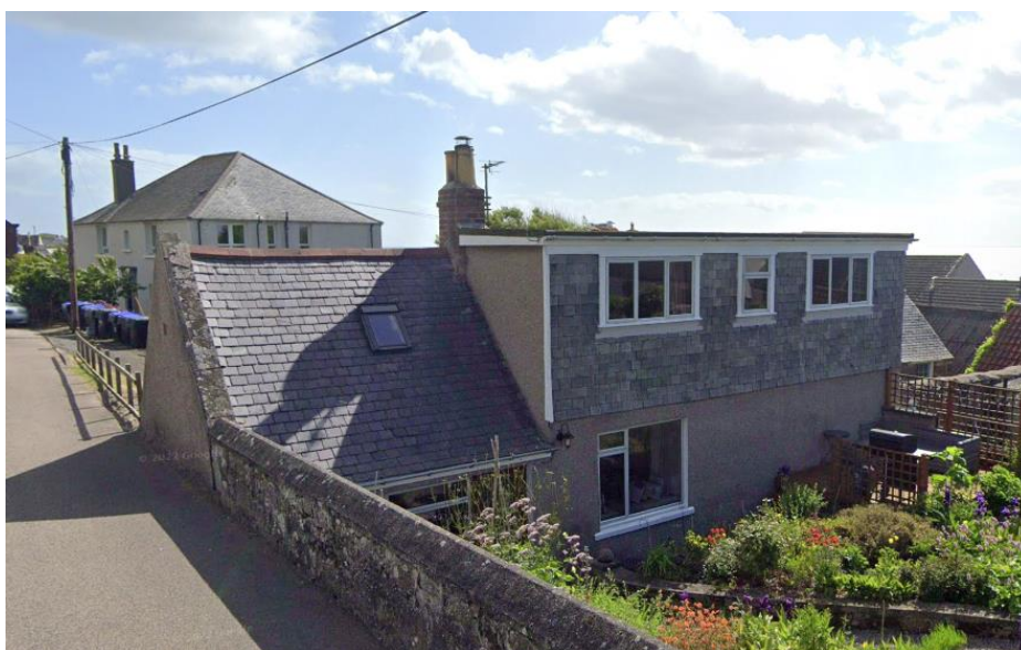
20 Main Street, Flat Roof with Membrane, White uPVC Windows - Note also the rooflight.
