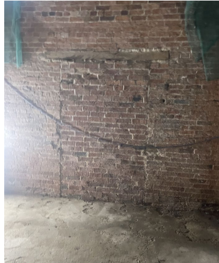
Plate 11: Interior view of blocked opening on west elevation proposed to be reopened.
