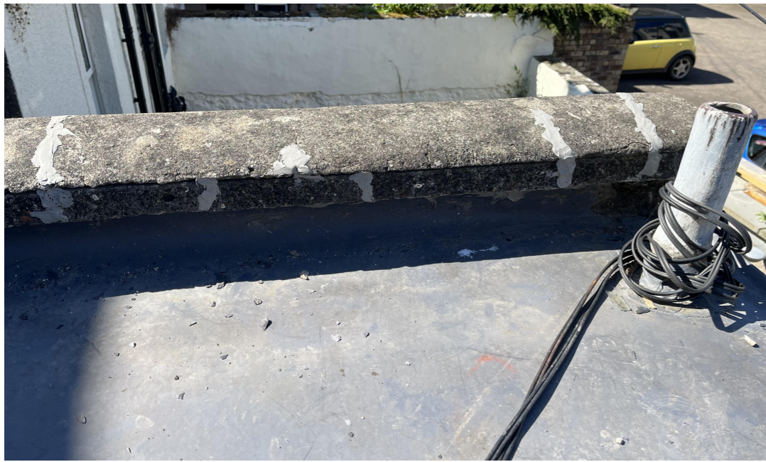
Before Single ply roof membrane, established as source of the leak, not ragged into rendered wall
