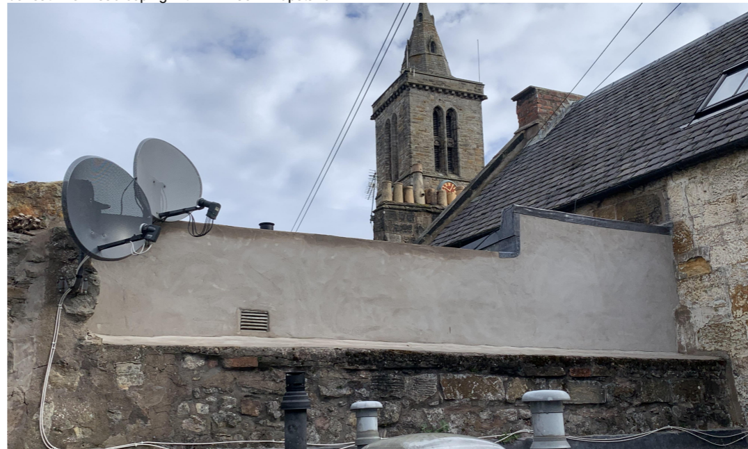
After New render finish to existing wall, similar to existing, lead coping on wall by bathroom
