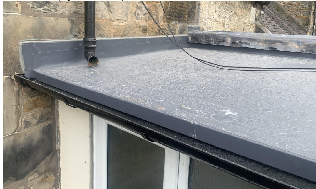
After New single ply roof membrane to match existing, ragged into wall and beneath new lead coping with min 150mm upstand.
