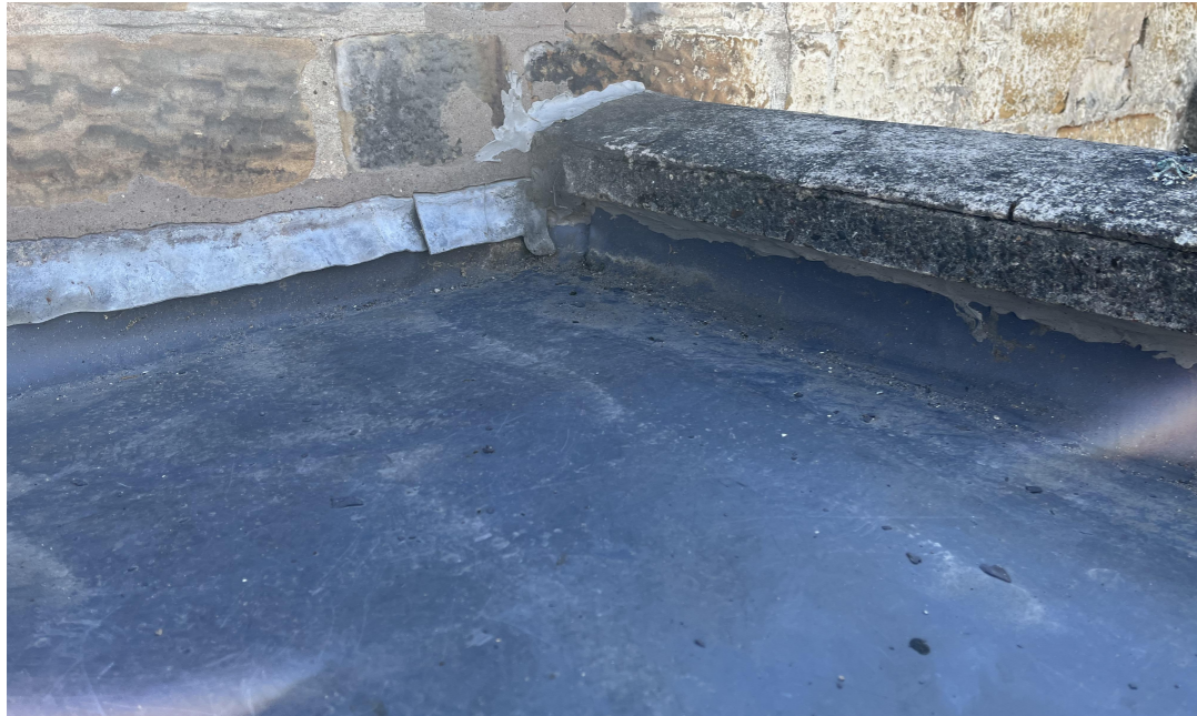
Before Single ply roof membrane, established as source of the leak, not ragged into rendered wall
