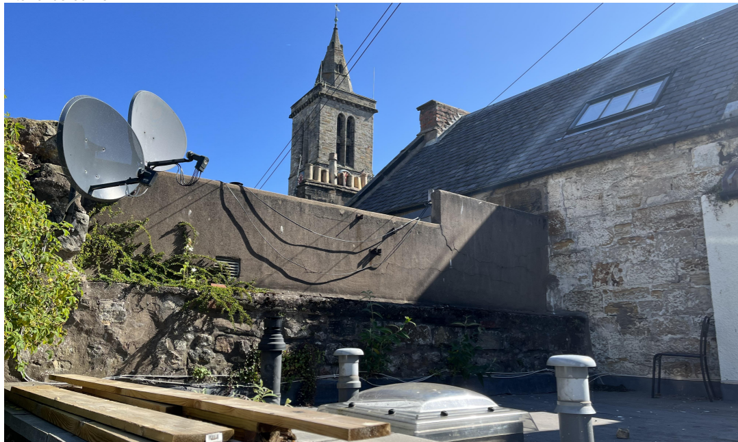
Before Render finish to wall showing cracking
