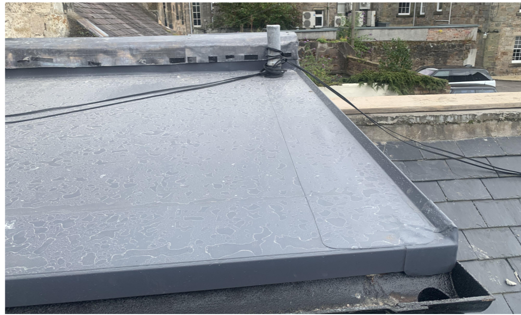
After New single ply roof membrane to match existing, ragged into wall and beneath new lead coping with min 150mm upstand.
