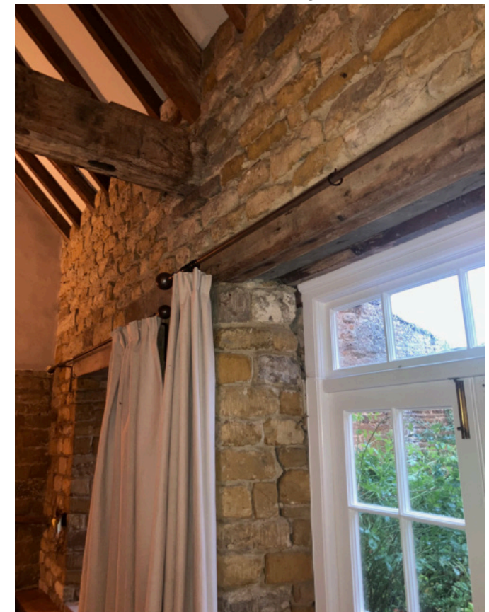
Existing Deteriorating External Door Opening
