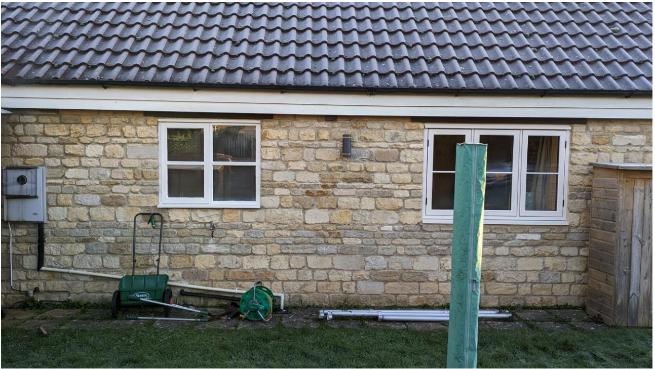
Photograph showing the western elevation and the window (lefthand side) to be replaced by an entrance door.
