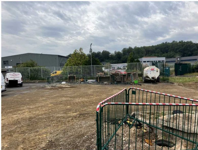
Pic 5 shows a view looking across the proposed development site whilst site clearance works were underway, with the existing site entrance centre right of the picture.
