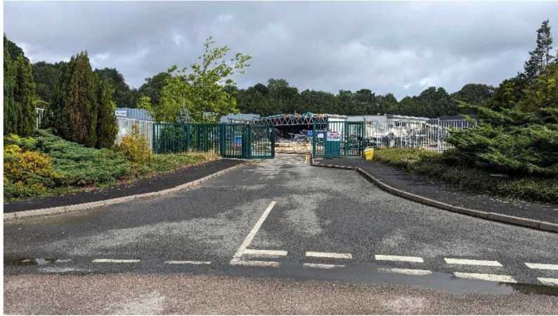
Pic 3 shows a view looking north from Chapman Way towards the existing proposed development site entrance whilst demolition works were underway.
