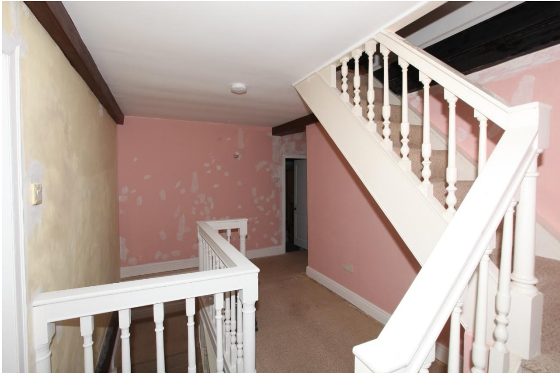
Illus. 21. The stair landing from the east, with the attic stair on the right. As elsewhere in the building, the few exposed structural timbers consist of pine in a manner that only became the norm at the end of the 18 th century. The staircase has been much altered but may retain some old elements and is in keeping with the character of the facade.
