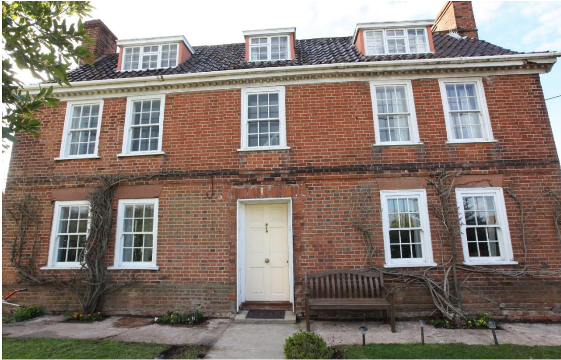
Illus. 3. The Flemish Bond brickwork of the facade has been heavily repointed, obscuring the evidence of its original arrangement, but in all probability it was identical to that shown in figure 8-10. The area between and around the four left-hand windows was rebuilt when the unusual adjoining sashes were separated. All but the penultimate first-floor window on the right contain horns and cannot pre-date the mid-19 th century (i.e. the sides of their upper sashes project beneath their lower rails to strengthen the joints in a manner not seen before this date).
