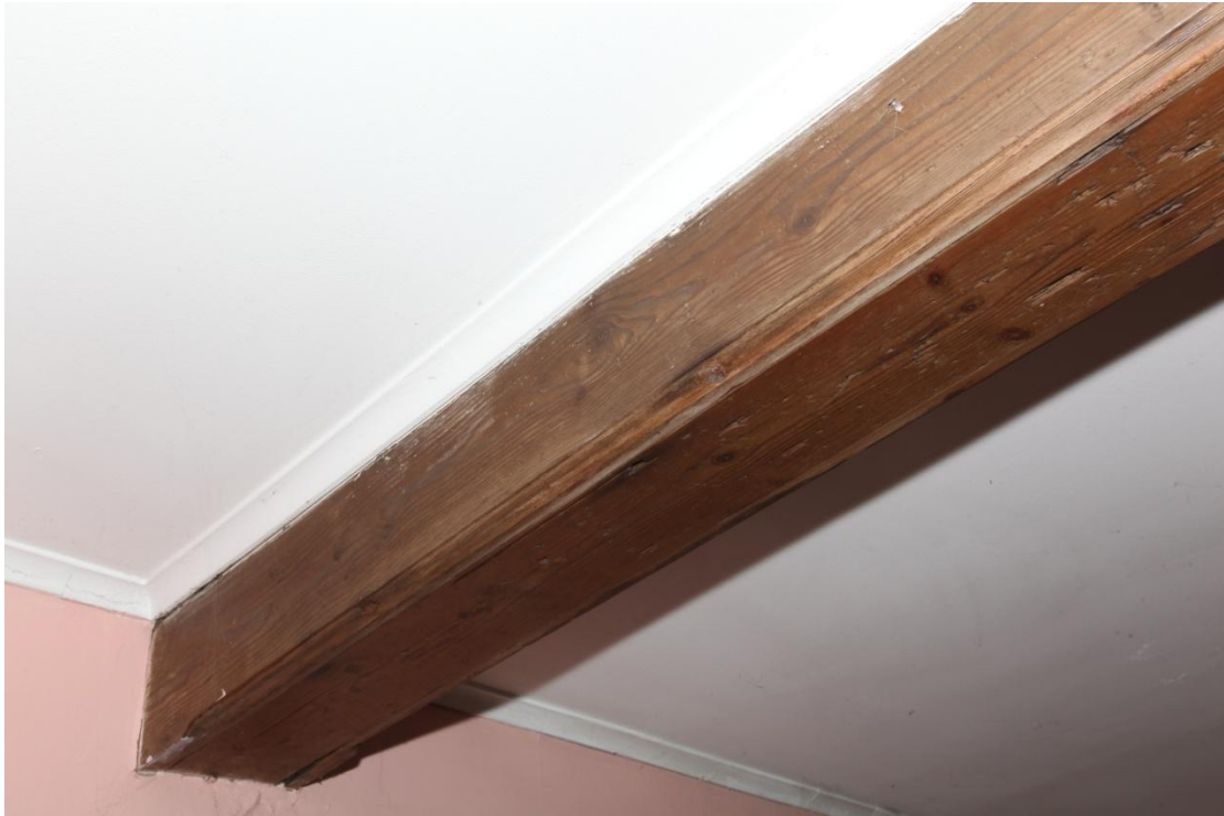
Illus. 19. A detail of the binding joist in the dining room (illustration 18), which is hidden by chamfered pine boards. These timbers are of some age, with chamfers that respect the width of the building, and may be original to the structure.
