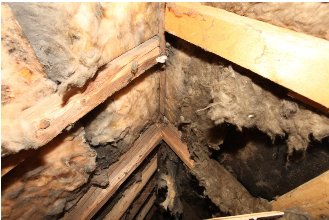
Illus. 26. The apex of the roof structure showing its pine rafters nailed to an ostensibly original ridge-board interrupted by a principal truss in the centre. The larger principal rafters are secured by a peg. The use of pine and a ridge board in this way is unlikely to pre-date the end of the 18 th century and is more typical of the early-19 th century.
