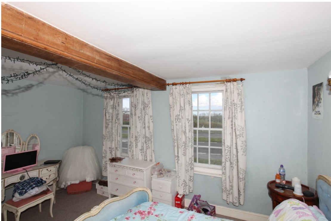
Illus. 24. The front wall of bedroom 2, which is divided from the rear corridor by a late-20 th century partition. The binding joist on the left retains what may be its original moulded pine boards.
