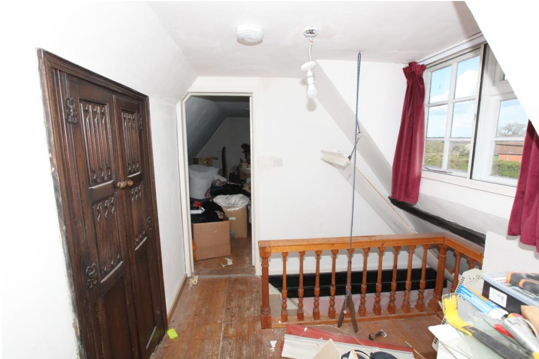
Illus. 25. The modern stained pine stair balustrade on the attic landing, with a built-in ‘Old Charm’ mid-20 th century cupboard door on the left. The structure is largely hidden at this level by the plasterboard of a late-20 th century refurbishment, but the original rafters are visible above the ceiling (illustration 26). The horizontal timber beneath the window may represent an original butt-purlin.
