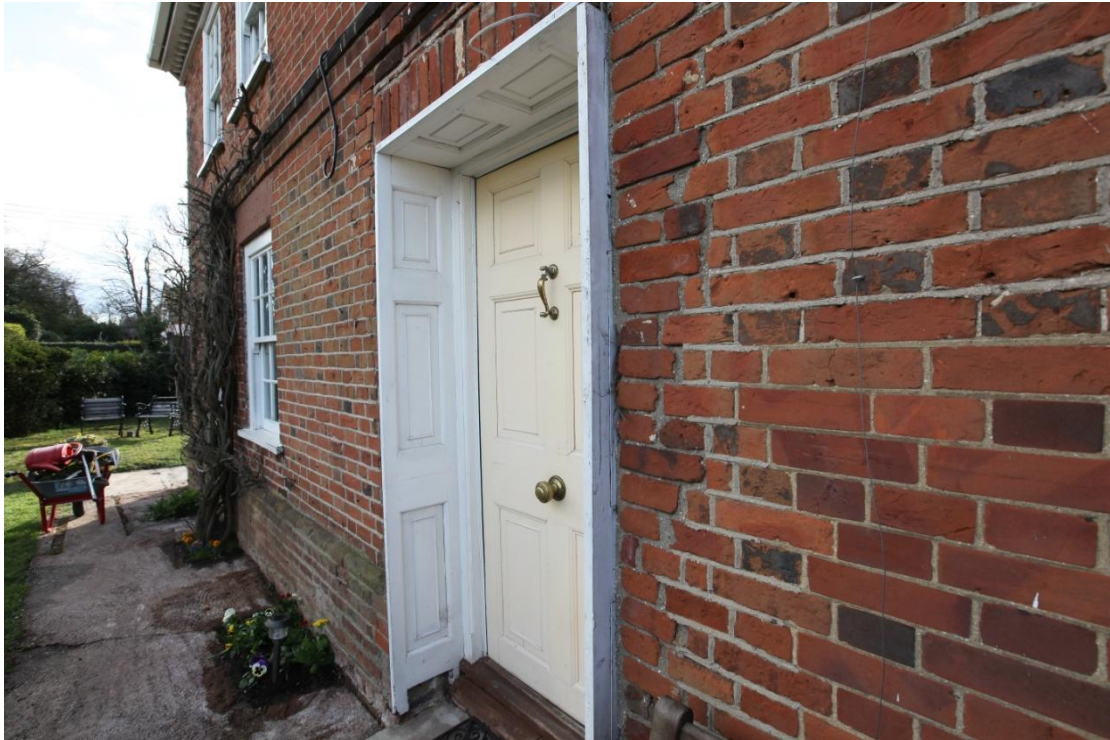
Illus. 5. A further detail of the main entrance showing the extent to which the panelled door surround projects beyond the wall face. Although dating from the 19 th century this panelling is not shown in the early-20 th century images and does not fit the building. It is likely to have been installed by the previous owner who is understood to have been a professional furniture restorer, and given the building's complex history as a Post Office and a pair of low-status cottages any potentially original fixtures and fittings should be treated with similar caution.
