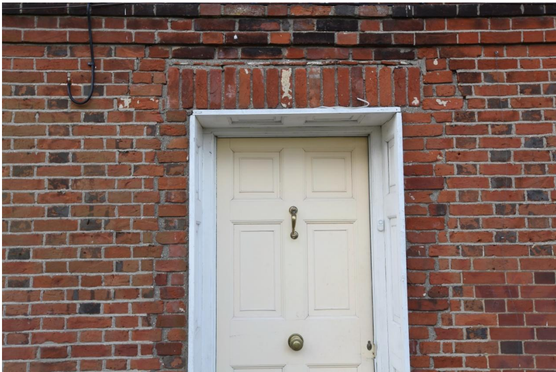
Illus. 4. A detail of the central entrance which is defined by recent brickwork laid in hard grey cement mortar with a crude modern flat arch above. The Post Office entrance may have been widened at some point, and the flat arch replaced a Georgian flat hood.
