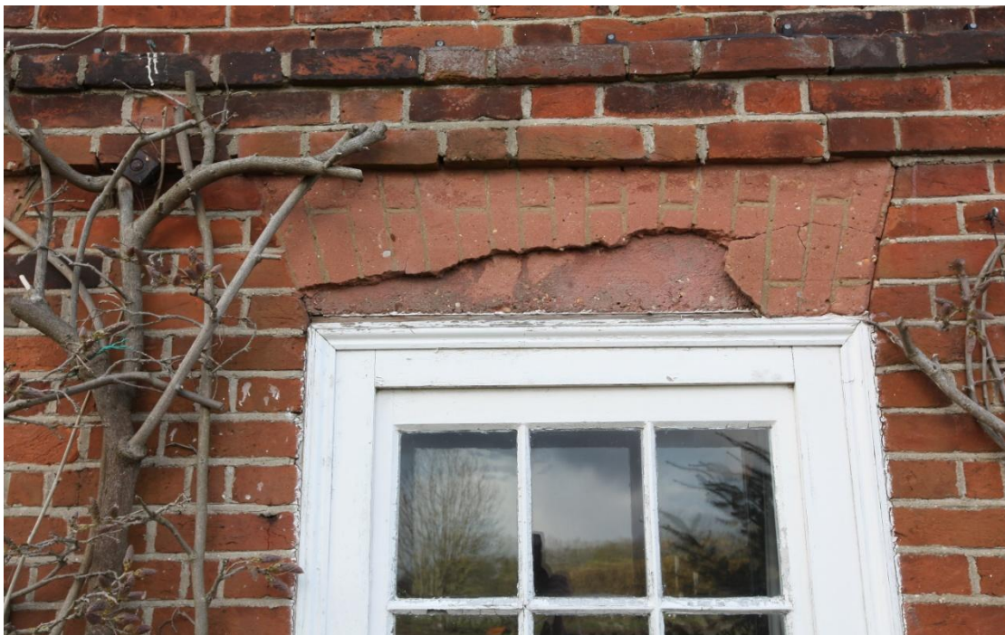
Illus. 6. A detail of the apparent flat arch over the right-hand ground-floor window which in fact consists of a concrete lintel covered by a recent layer of cement incised and painted to resemble brickwork. The other three arches are identical.
