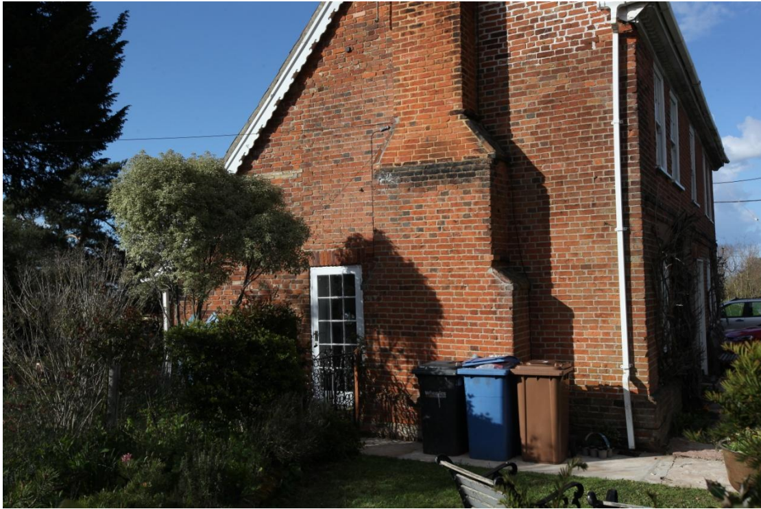
Illus. 7. The modern glazed door in the southern gable is respected by an ostensibly 19 th century flat arch and occupies the position of the entrance to the blacksmith's cottage in figures 8-10. The brickwork of the rear lean-to on the left is modern and replaced the render shown in the early photographs.
