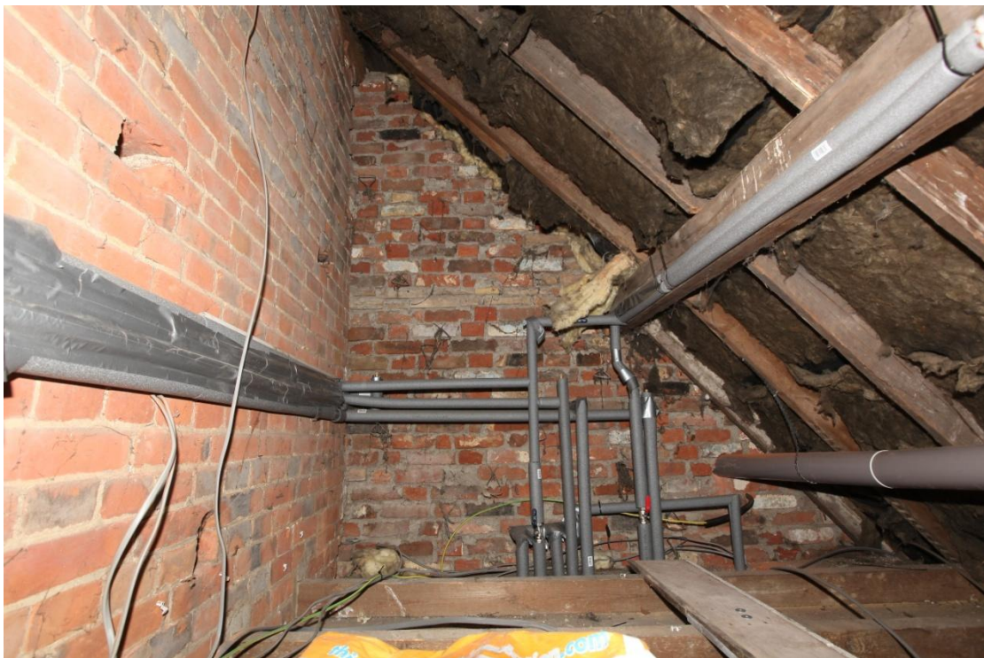
Illus. 12. The internal southern roof gable of the single-storied lean-to in illustration 11, with the original rear wall of the house on the left. The gable consists of re-used brick laid in cement mortar and dates only from the 20 th century. The original rear wall lacks windows and evidently adjoined a similar timber-framed lean-to from the outset.
