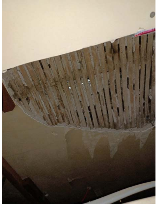
Photograph 4 – Example of missing plaster to lath and plaster ceiling over main retail space
