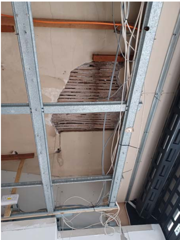
Photograph 9 – Area of failed plaster
