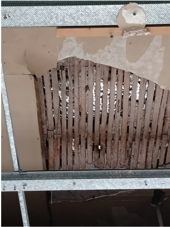
Photograph 7 – Area of failed plaster
