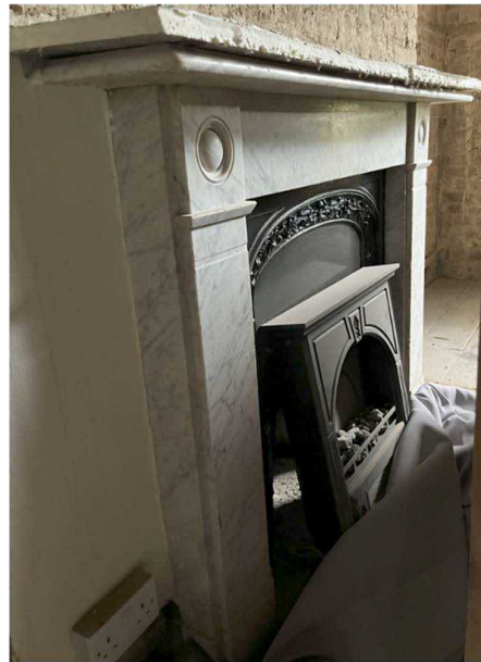
Cast iron fireplaces with marble surrounds.
