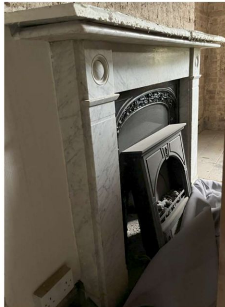
Cast iron fireplaces with marble surrounds.
