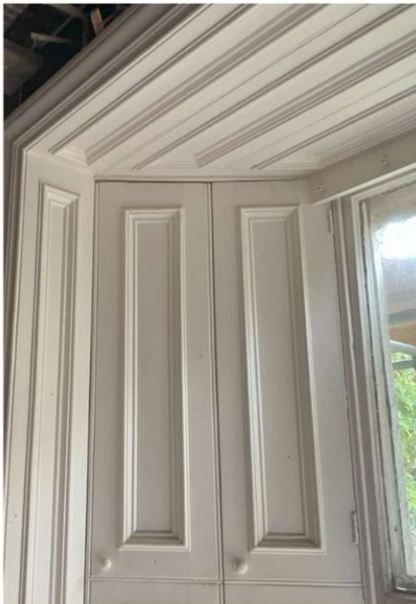
Wood panelling and shutters around windows and doors at rear of ground floor.
