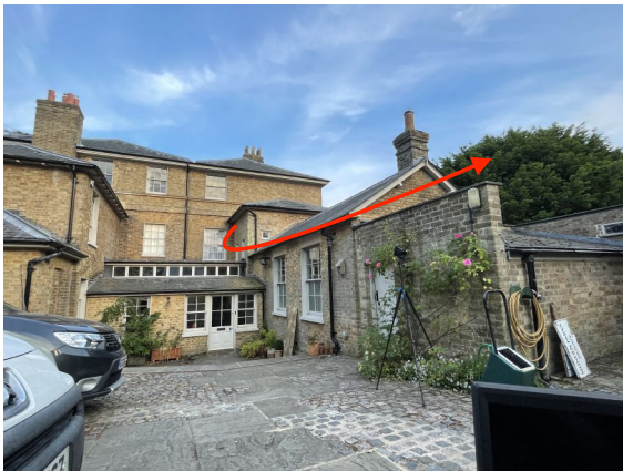
Roost C | 2 Common pipistrelles emerged from a gap in the eaves on the northern elevation of the property.
