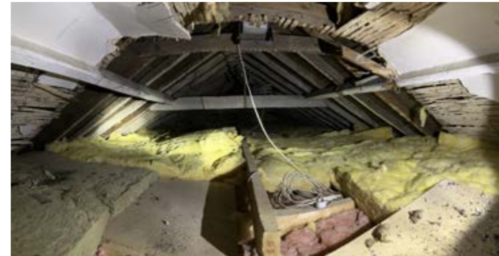
Fig 11, the attic above the mission room, remains of original vaulted ceiling
