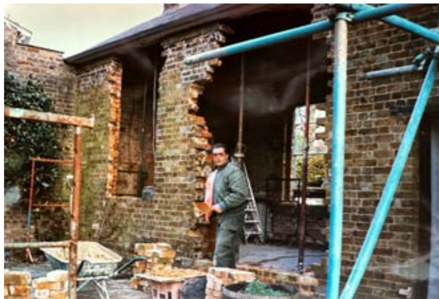
Fig 10 Patio doors removed, new window openings formed, interior stripped back to bare bricks, c.1995
