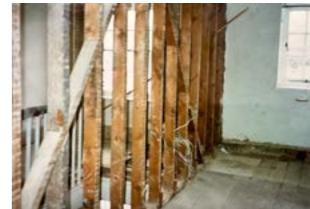
Fig 6 original wall adjacent to the staircase being removed c.1995 The window on the right was enlarged in the 1990s to match the sash on the left
