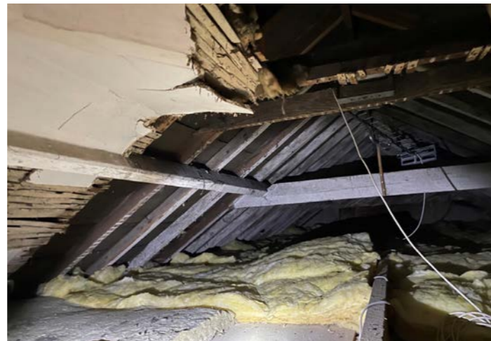
Photos taken above non-original ceiling line, showing the original ceiling form, and location of roof structure. The proposal looks to reinstate the original room (assumed Mission Room) proportions.
