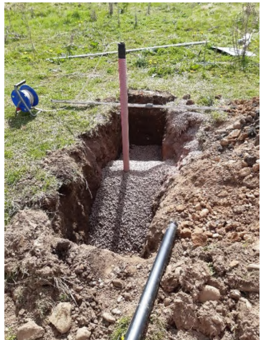
SA01 Soakaway set up.
