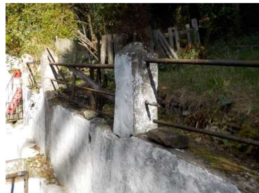
Existing guarding to the top of the retaining wall Current guarding does not meet current safety standards
