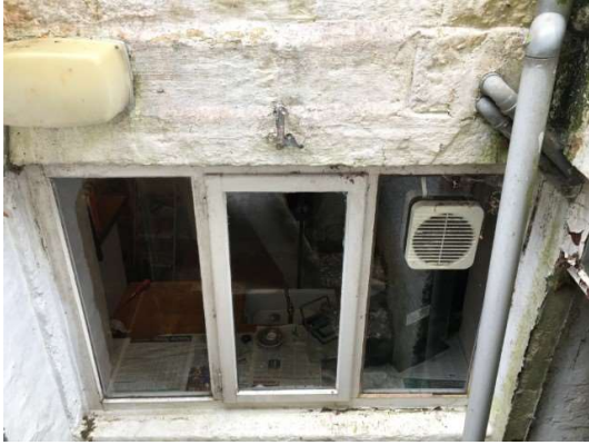
Existing external light
