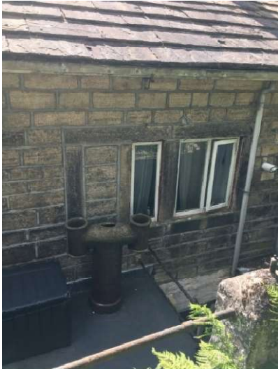
Proposed location for new door opening (external) The proposed new door would open on to the flat roof of the single-storey offshot
