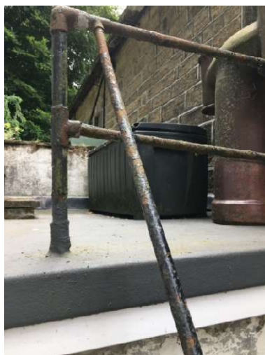
Existing guarding to the open edge of the offshot Current guarding does not meet current safety standards
