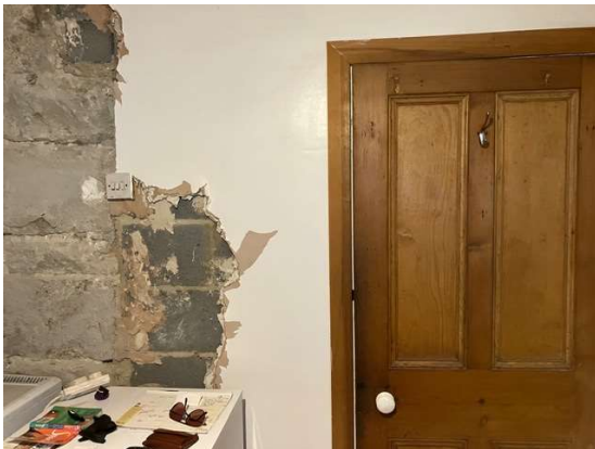
Existing opening between living room and kitchen (seen from kitchen side) showing modern blockwork infill to left hand side of door
