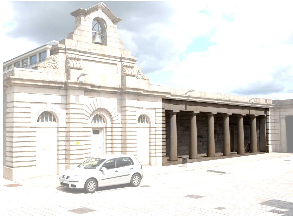
Fig. 3: Canopy with doric columns, prior to any works undertaken at the yard
