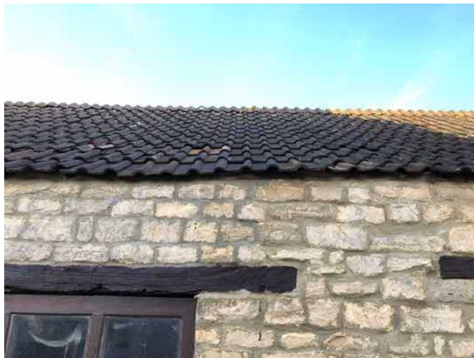
Photograph 6: Barn – gaps under tiles and ridge tiles providing direct access to the interior (April 2018).
