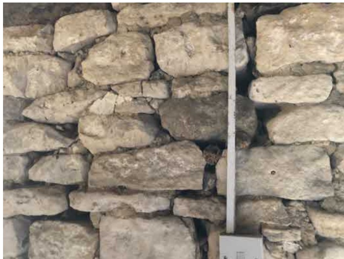
Photograph 11: Barn – gaps in interior walls (April 2018).
