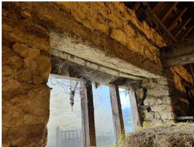
Photograph 9a: Barn – gap in timber lintel above window – heavily cobwebbed and no evidence of use (December 2023).
