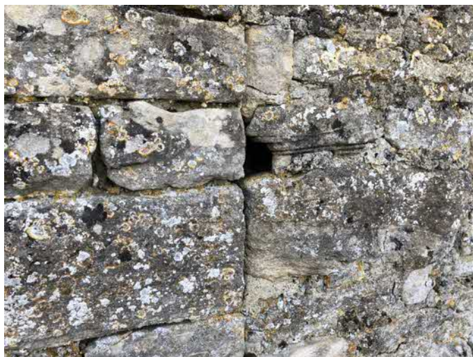
Photograph 7: Barn – one of a small number of holes in the external walls (April 2018).
