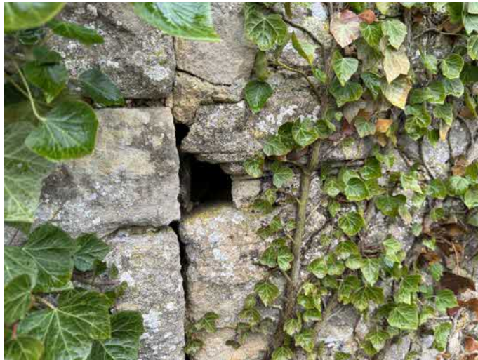
Photograph 7a: Barn – one of a small number of holes in the external walls (December 2023).
