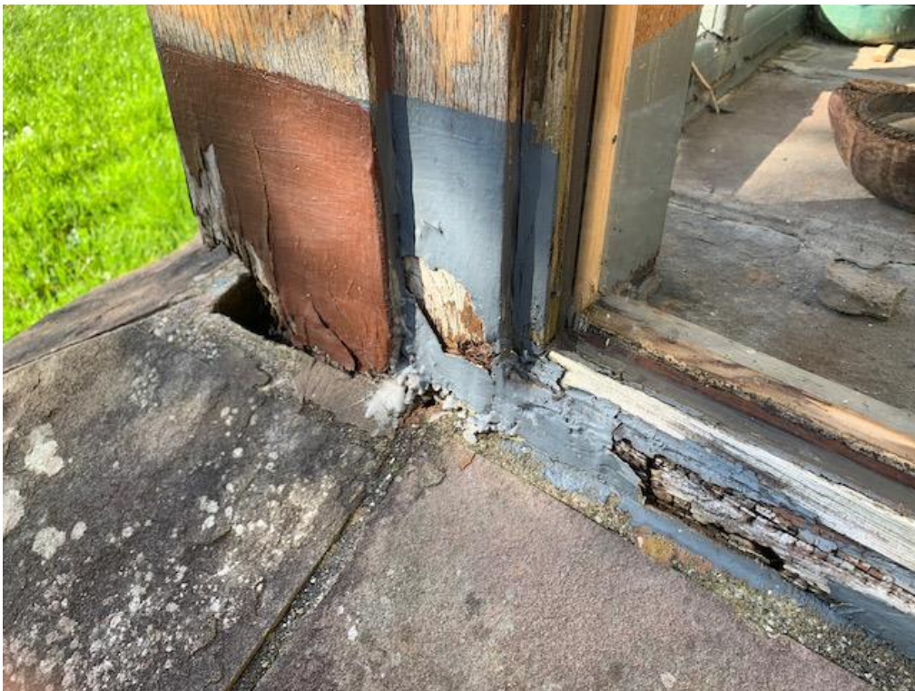
Figure 2 - typical condition of conservatory
