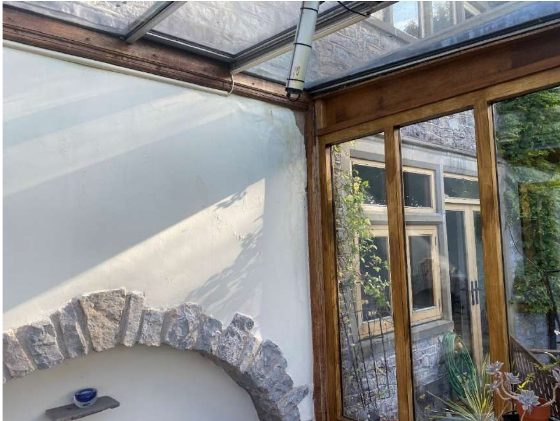
Photograph 13 – Signs of damp present
