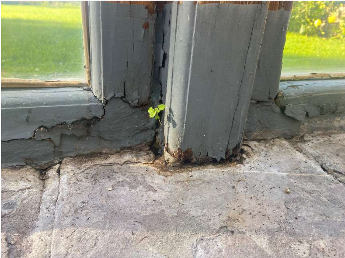
Photograph 9 – Rotten timber at bottom of post
