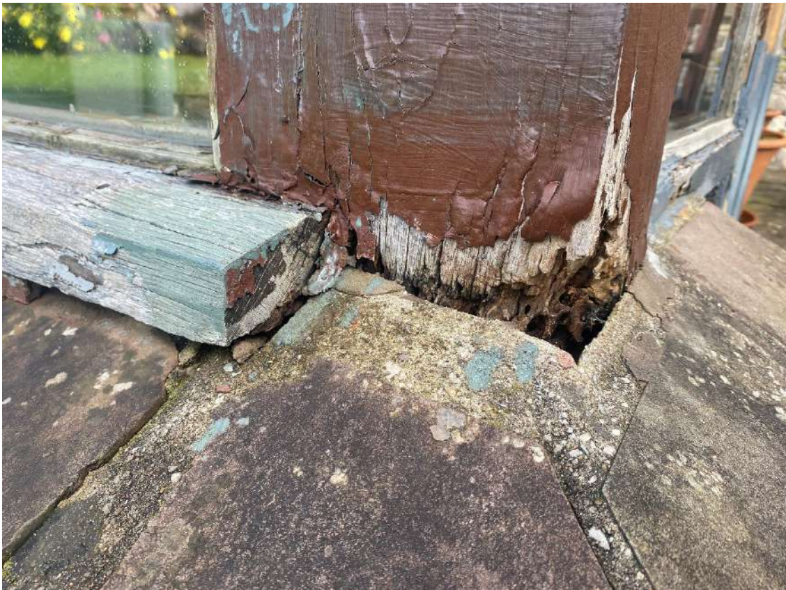
Photograph 8 – Rotten timber at bottom of post
