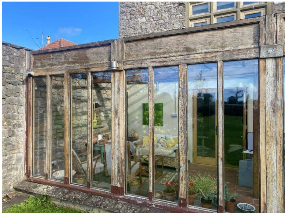
Photograph 14 – Discoloration in timber shows protective layer diminished
