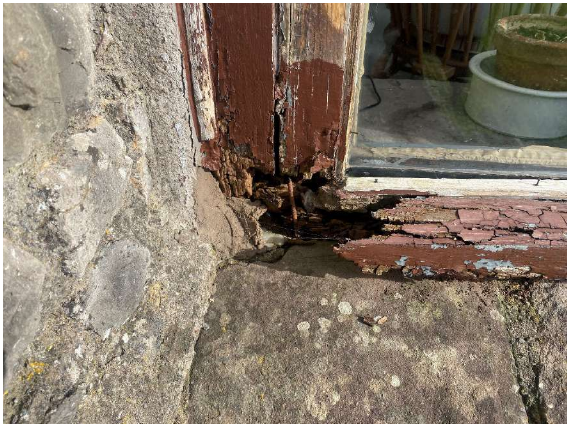
Photograph 10 – Rotten timber at base of frame
