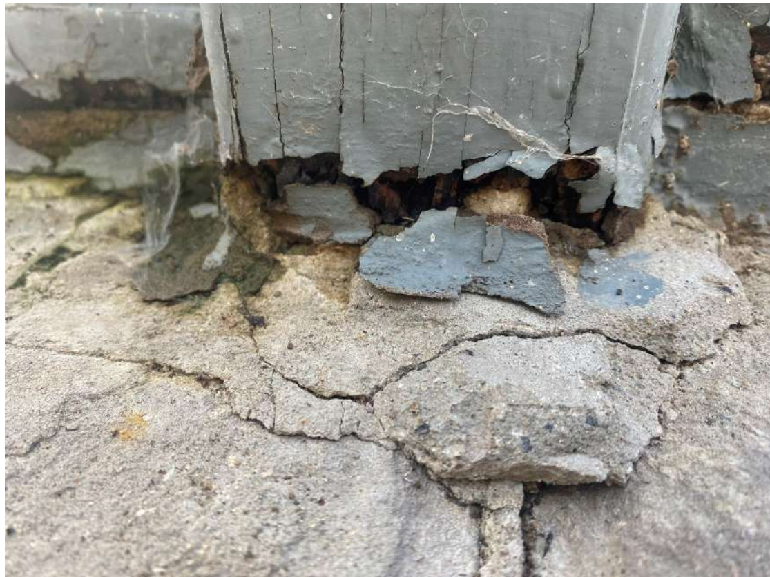
Photograph 6 – Rotten timber at bottom of post
