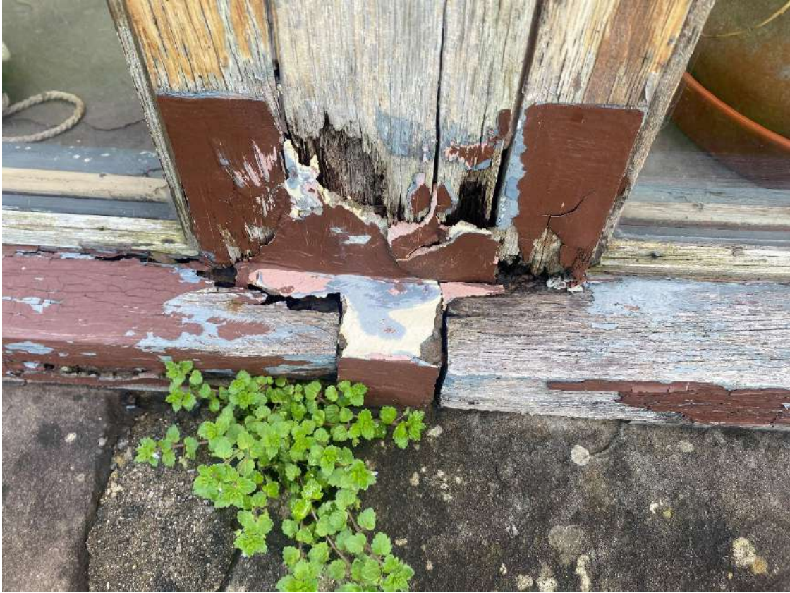
Photograph 7 – Rotten timber at bottom of post
