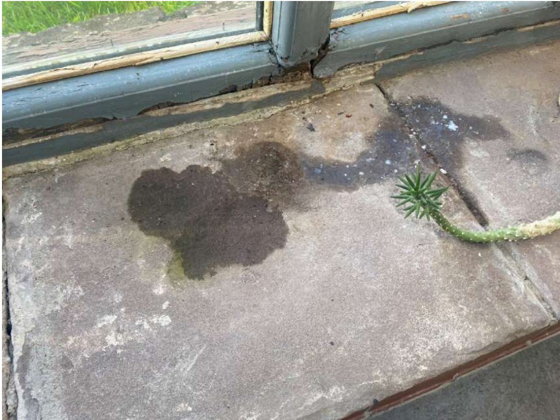
Photograph 11 – Rotten timbers and signs of water ingress
