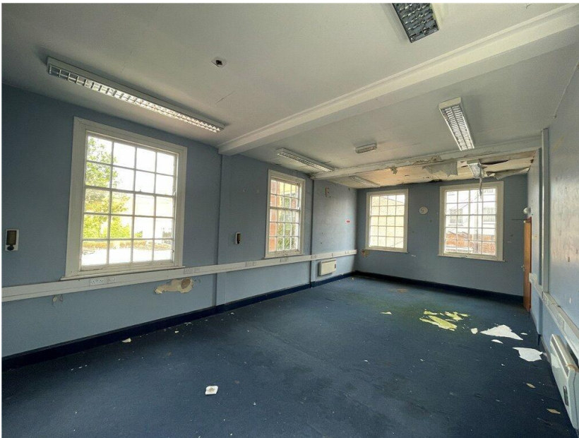
Figure 5 – photo showing large windows giving ample natural light to what would be flat 6. As the building is vacant and being regularly vandalised most of the windows are currently boarded up.
