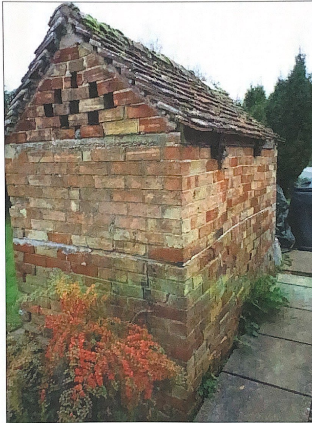
Former privies in poor condition
