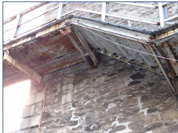
Gantry fixed to wall and bird nest
