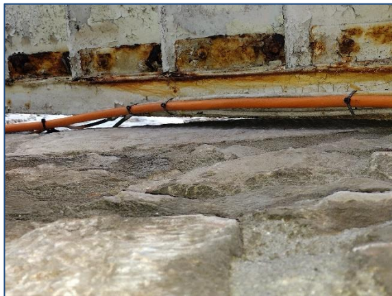
Large gap behind gantry
