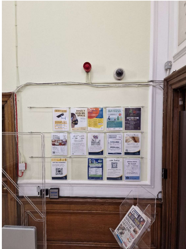
GF - Existing - Old CCTV Camera Location In Lobby SE Corner - To be Removed (Not on Plans)
