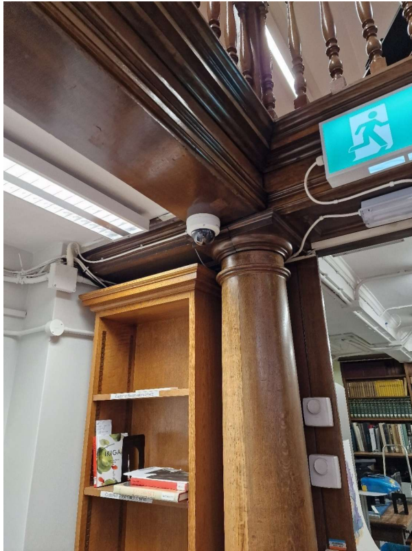
GF - Existing - Old CCTV Camera Over Desk - To be Removed (Not on Plans)
