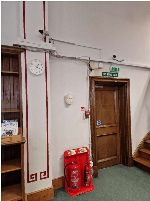
1F - Existing - 2no. Old CCTV Cameras On North Wall - To be Removed (Not on Plans)
