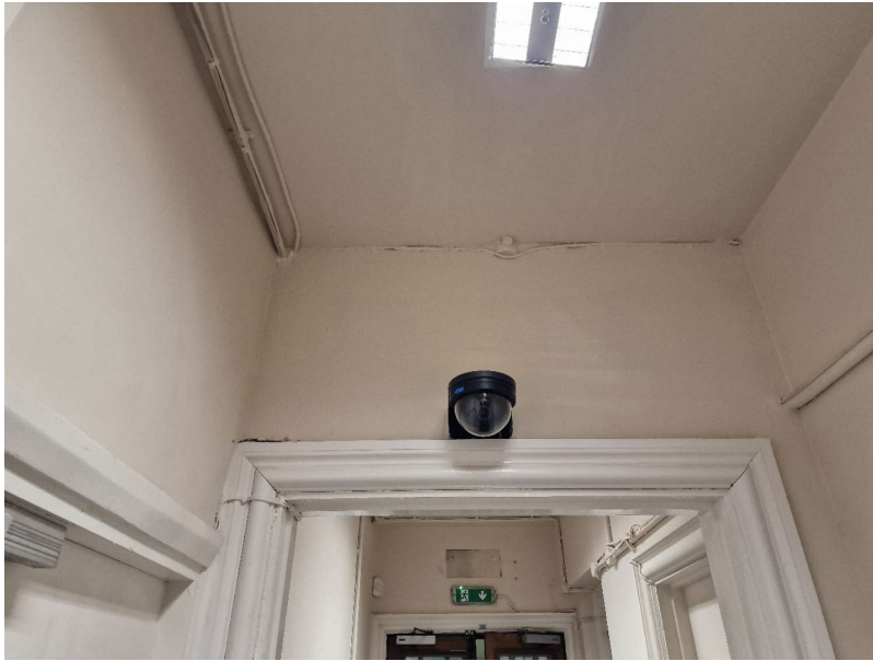
2F - Existing - CCTV To Library Work Area North Exit - To be Removed (Not on Plans)
