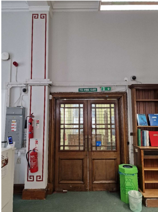
1F - Existing - 2 No. CCTV Cameras Around Entrance Doors - To be Removed (Not on Plans)
