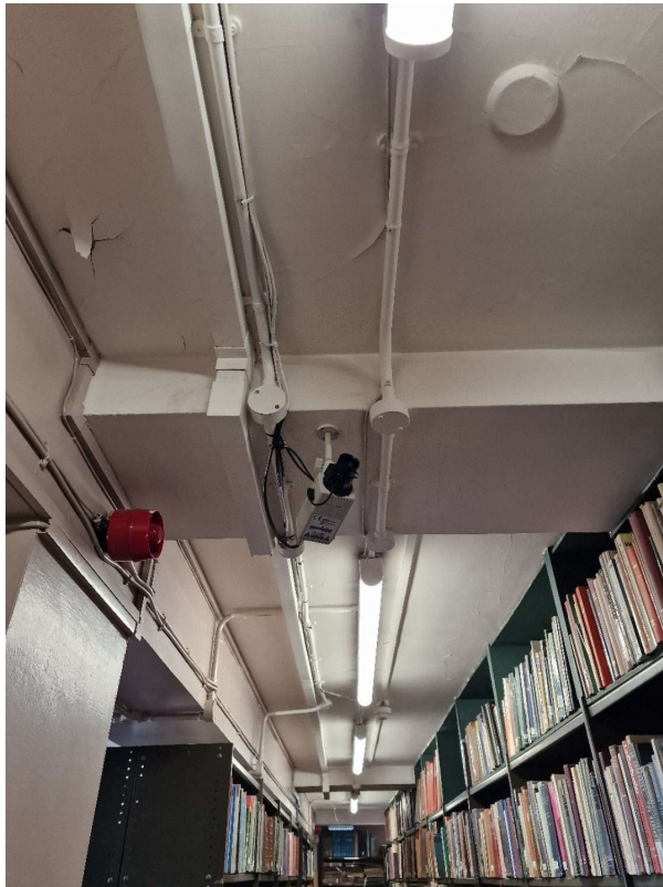
2F - Existing - Old CCTV Camera To Book Store Ceiling - To be Removed (Not on Plans)
