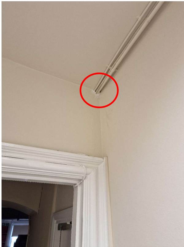
2F - Proposed - New CCTV Camera For Circulation Exit
