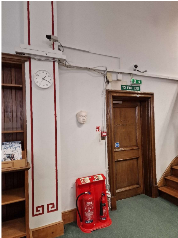
1F - Existing - 2no. Old CCTV Cameras On North Wall - To be Removed (Not on Plans)
