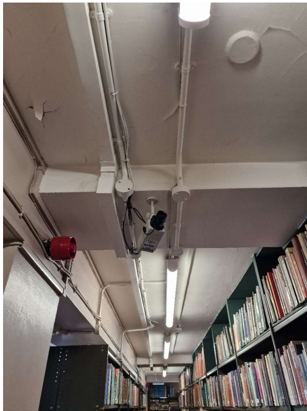
2F - Existing - Old CCTV Camera To Book Store Ceiling - To be Removed (Not on Plans)
