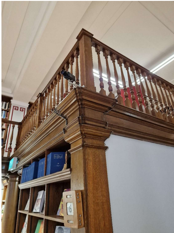
GF - Existing - Old CCTV Camera On NE Balcony Corner - To be Removed (Not on Plans)
