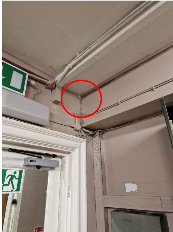
2F - Proposed - New CCTV Camera To Book Storage NE Corner
