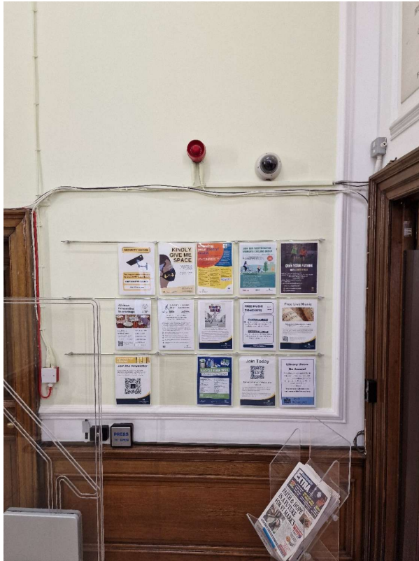
GF - Existing - Old CCTV Camera Location In Lobby SE Corner - To be Removed (Not on Plans)
