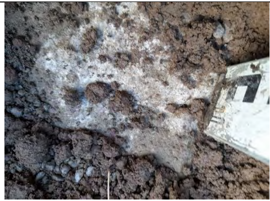
Photograph 12: View of soil within cover system and geotextile at base in front of Plot 38.
