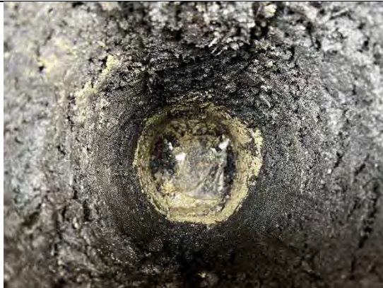
Photograph 115: View of soil within cover system and geotextile at base in front of Plot 53.
