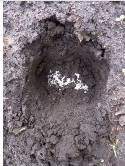
Photograph 186: View of soil within cover system and geotextile at base of shared soft landscaping B3.
