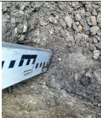
Photograph 39: View of soil within cover system and geotextile at base in front of Plot 41.
