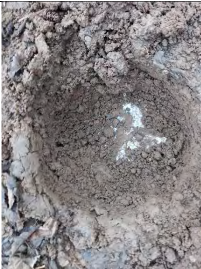
Photograph 189: View of soil within cover system and geotextile at base of shared soft landscaping B4.
