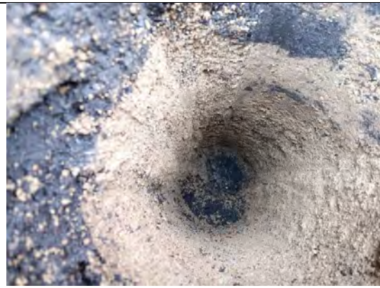
Photograph 78: View of soil within cover system and geotextile at base in rear of Plot 46.
