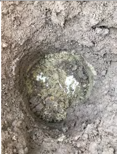
Photograph 177: View of soil within cover system and geotextile at base of shared soft landscaping A3.
