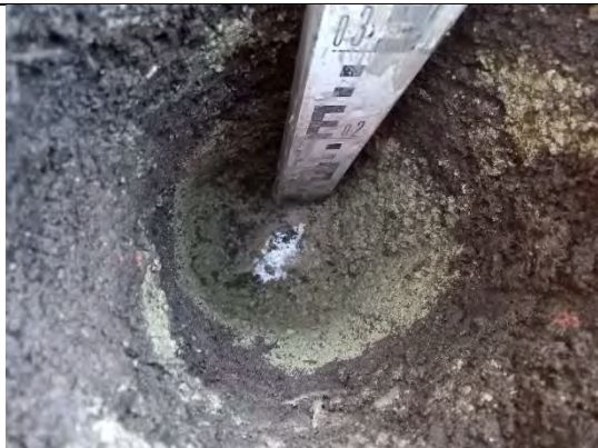
Photograph 195: View of soil within cover system and geotextile at base of shared soft landscaping C2.
