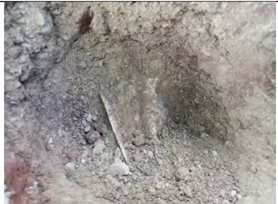
Photograph 36: View of soil within cover system and geotextile at base in rear (S) of Plot 40.
