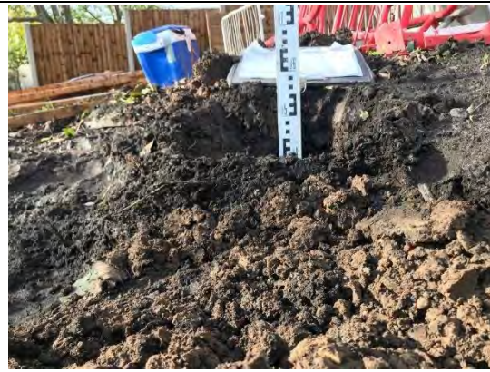
Photograph 5: View of depth of soil within the rear (N) garden of Plot 37.
