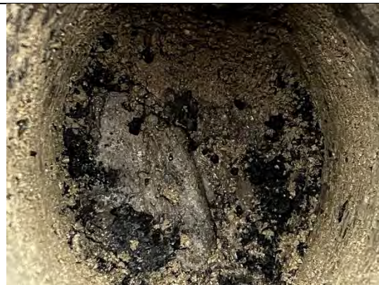
Photograph 145: View of soil within cover system and geotextile at base in rear of Plot 58.
