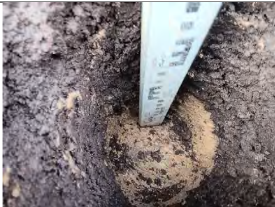
Photograph 87: View of soil within cover system and geotextile at base in front of Plot 48.
