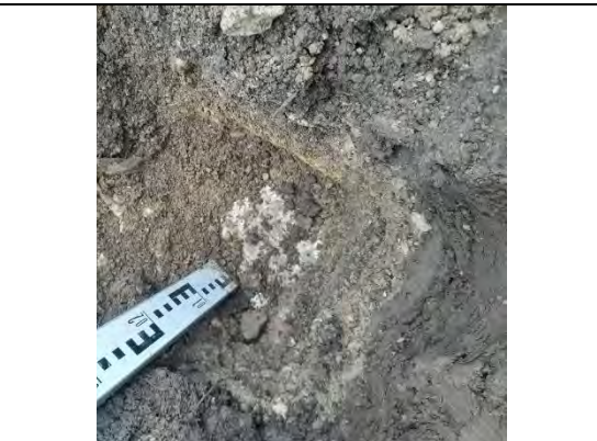
Photograph 48: View of soil within cover system and geotextile at base in front of Plot 42.
