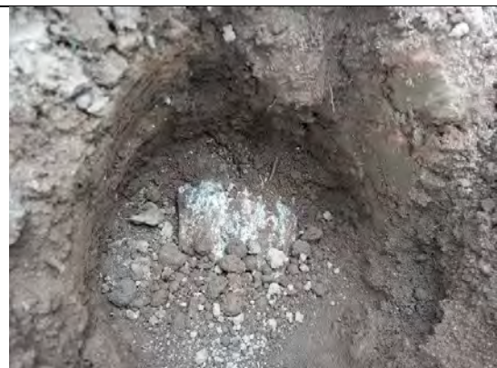
Photograph 24: View of soil within cover system and geotextile at base in rear (S) of Plot 39.
