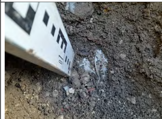
Photograph 21: View of soil within cover system and geotextile at base in front of Plot 39.
