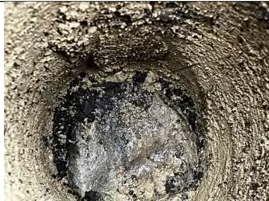
Photograph 139: View of soil within cover system and geotextile at base in rear of Plot 57.
