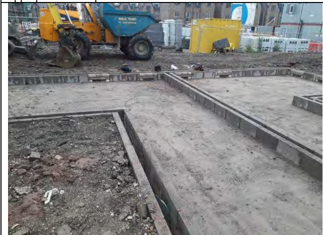
Photograph 5: Evidence of sub-floor void in Plot 45.
