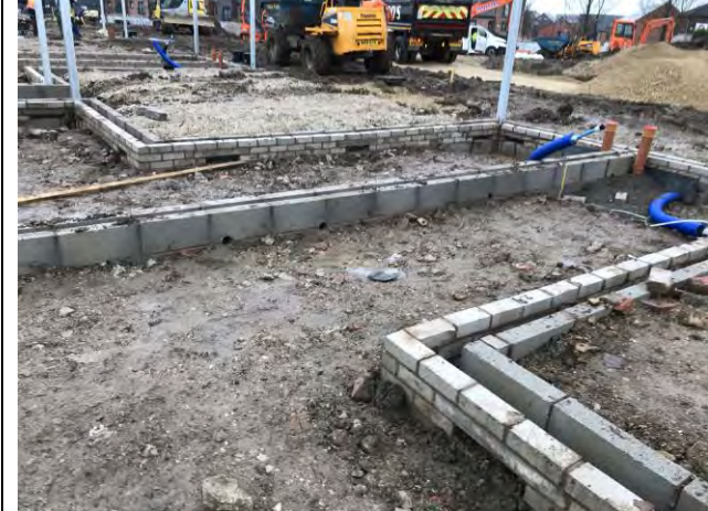
Photograph 5: Evidence of sub-floor void in Plot 50.
