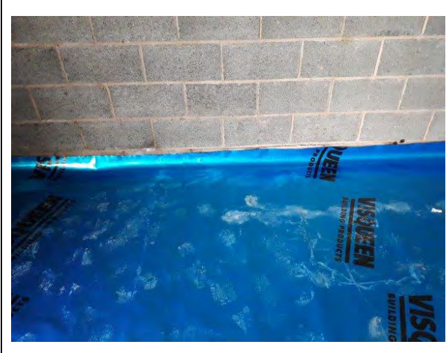
Photograph 3: Evidence of appropriate sealing of membrane to DPC with appropriate overlap for Plot 2.
