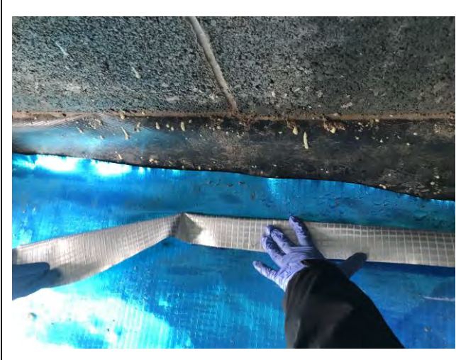
Photograph 3: Evidence of appropriate sealing of membrane to DPC with appropriate overlap for Plot 59.
