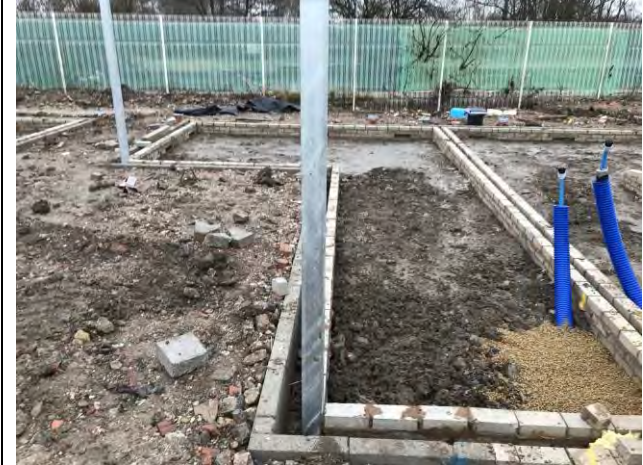
Photograph 5: Evidence of sub-floor void in Plot 59.
