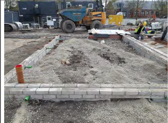
Photograph 5: Evidence of sub-floor void in Plot 9.
