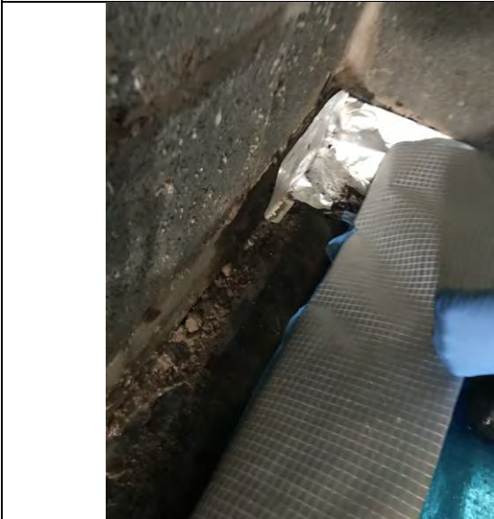
Photograph 3: Evidence of appropriate sealing of membrane to DPC with appropriate overlap for Plot 51.
