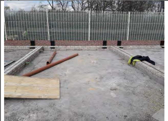
Photograph 5: Evidence of sub-floor void in Plot 8.
