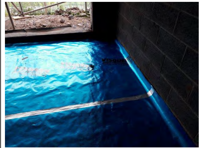
Photograph 3: Evidence of appropriate sealing of membrane to DPC with appropriate overlap for Plot 4.
