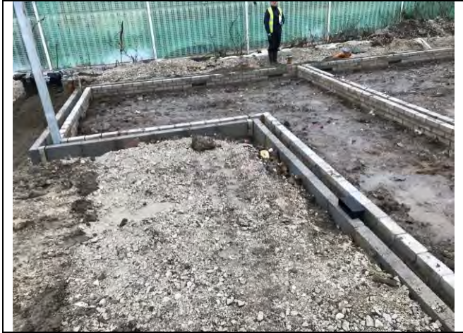
Photograph 5: Evidence of sub-floor void in Plot 55.
