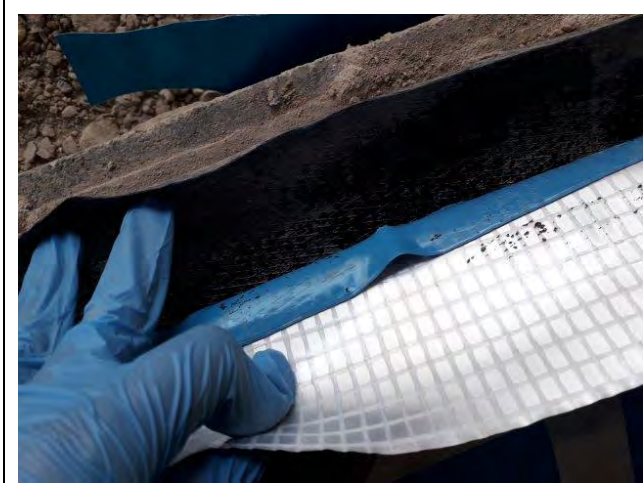
Photograph 3: Evidence of appropriate sealing of membrane to DPC with appropriate overlap for Plot 37.
