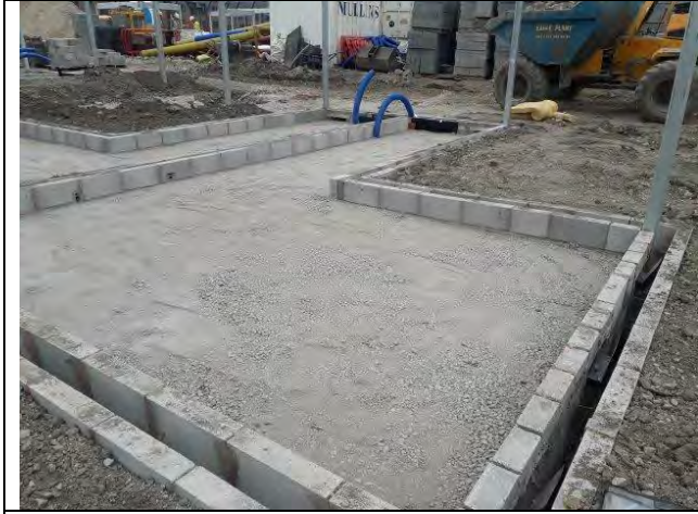
Photograph 5: Evidence of sub-floor void in Plot 37.
