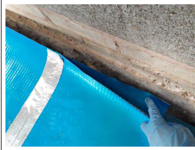
Photograph 3: Evidence of appropriate sealing of membrane to DPC with appropriate overlap for Plot 42.
