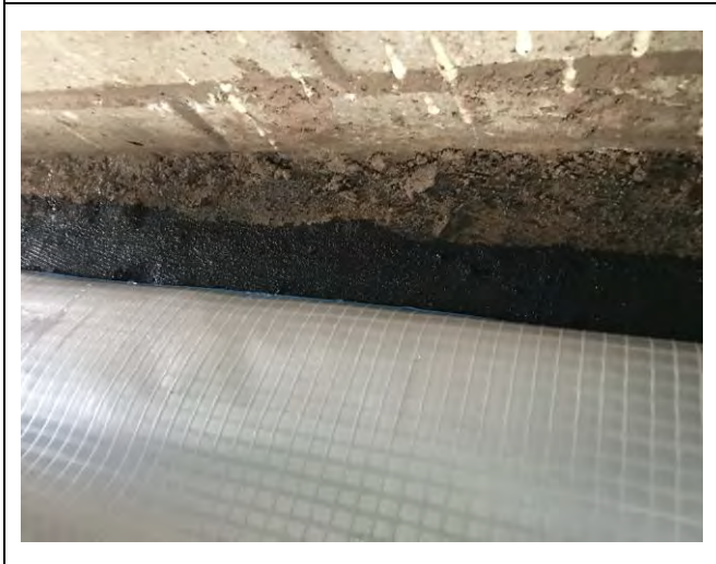
Photograph 3: Evidence of appropriate sealing of membrane to DPC with appropriate overlap for Plot 55.
