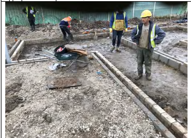
Photograph 5: Evidence of sub-floor void in Plot 57.
