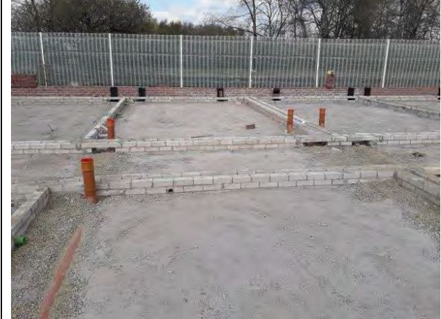
Photograph 5: Evidence of sub-floor void in Plot 3.
