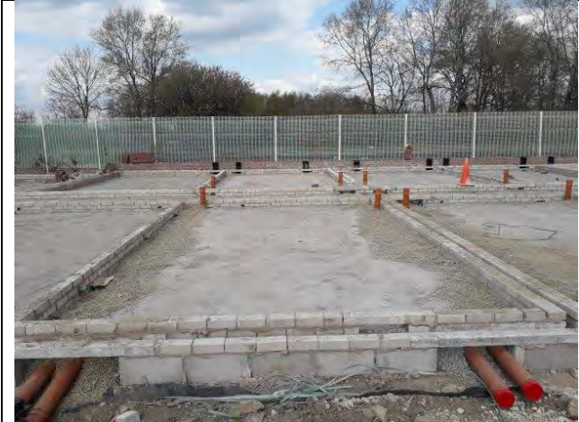
Photograph 5: Evidence of sub-floor void in Plot 4.
