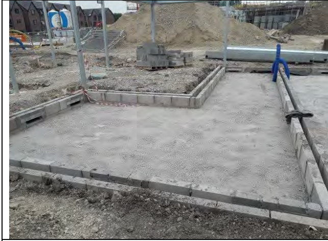
Photograph 5: Evidence of sub-floor void in Plot 42.
