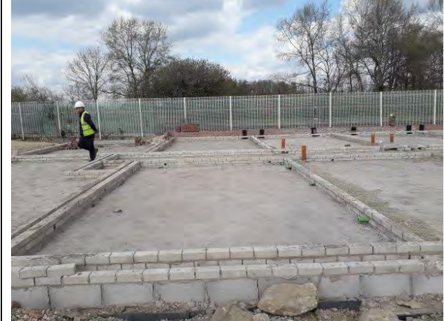
Photograph 5: Evidence of sub-floor void in Plot 1.
