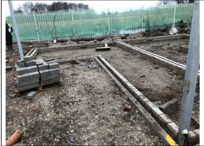
Photograph 5: Evidence of sub-floor void in Plot 52.
