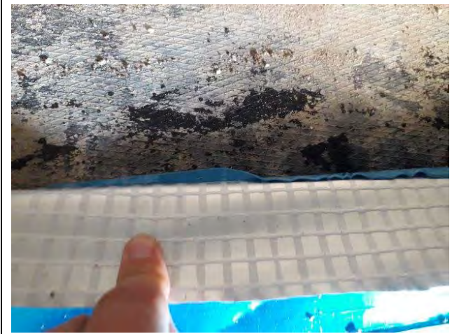
Photograph 3: Evidence of appropriate sealing of membrane to DPC with appropriate overlap for Plot 8.
