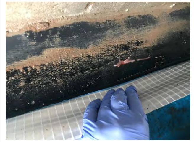
Photograph 3: Evidence of appropriate sealing of membrane to DPC with appropriate overlap for Plot 57.
