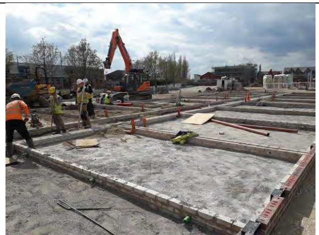
Photograph 6: Evidence of sub-floor void across apartment block.
