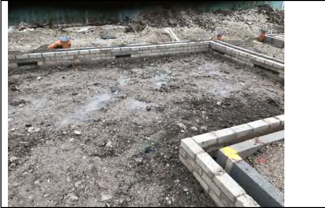
Photograph 5: Evidence of sub-floor void in Plot 56.
