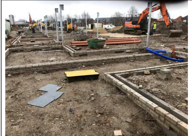
Photograph 5: Evidence of sub-floor void in Plot 49.
