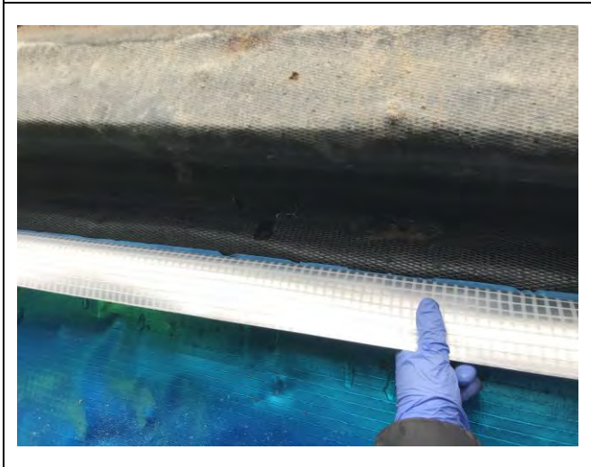
Photograph 3: Evidence of appropriate sealing of membrane to DPC with appropriate overlap for Plot 49.
