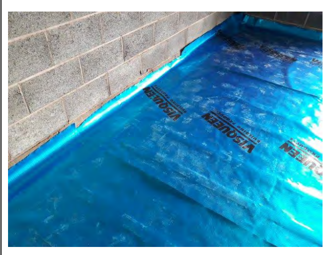
Photograph 3: Evidence of appropriate sealing of membrane to DPC with appropriate overlap for Plot 3.
