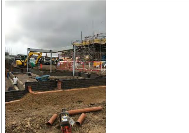
Photograph 5: Evidence of sub-floor void in Plot 61.
