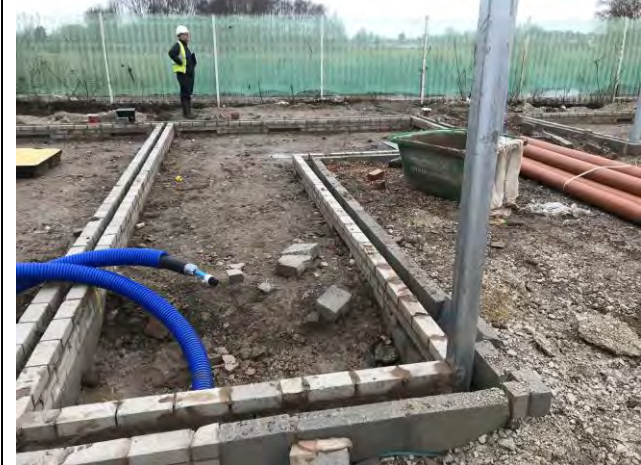
Photograph 5: Evidence of sub-floor void in Plot 51.
