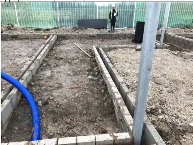
Photograph 5: Evidence of sub-floor void in Plot 54.
