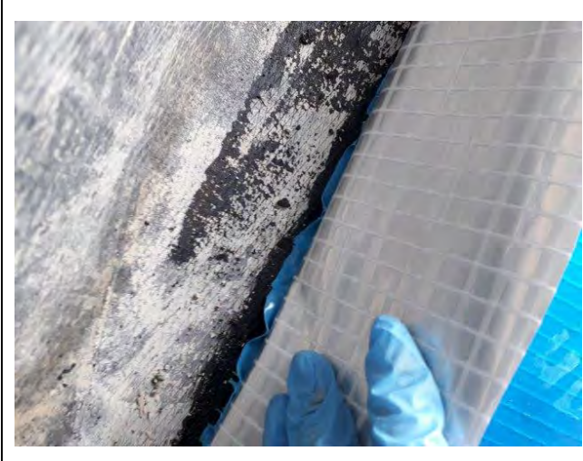
Photograph 3: Evidence of appropriate sealing of membrane to DPC with appropriate overlap for Plot 43.
