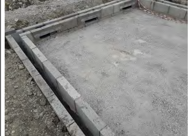
Photograph 5: Evidence of sub-floor void in Plot 43.
