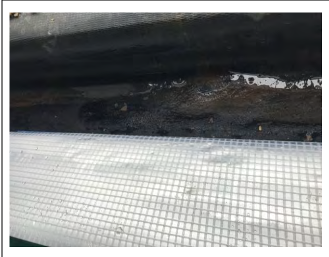
Photograph 3: Evidence of appropriate sealing of membrane to DPC with appropriate overlap for Plot 52.
