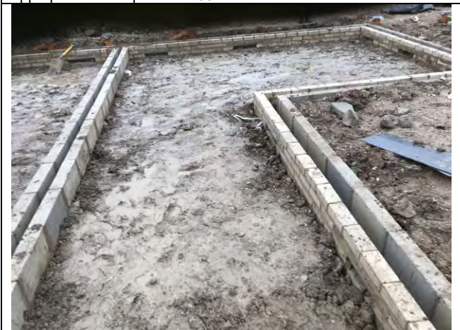
Photograph 5: Evidence of sub-floor void in Plot 58.
