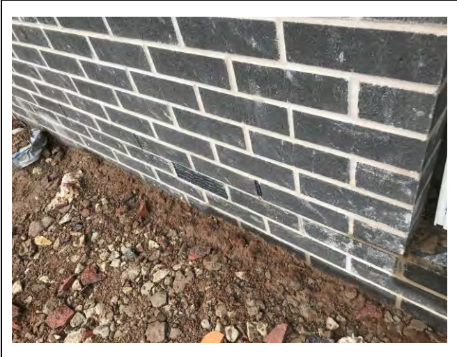
Photograph 3: Evidence of appropriate sealing of membrane to DPC with appropriate overlap for Plot 56.
