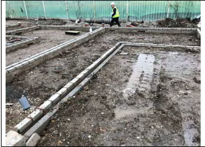
Photograph 5: Evidence of sub-floor void in Plot 53.
