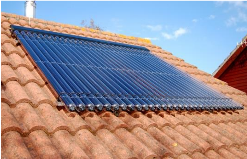
Figure 5: Typical solar thermal panel
