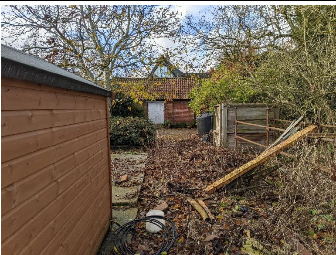
Photo 5 Area to the west of the PV array where the shallow dig cable route will be laid – looking west
