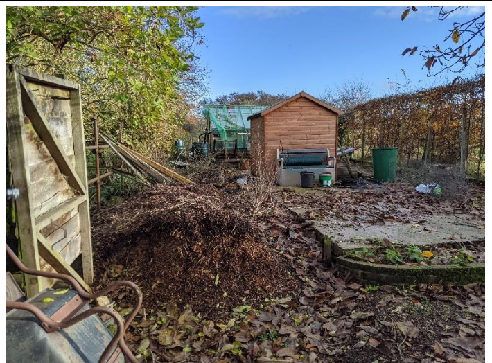
Photo 4 Area to the west of the PV array where the shallow dig cable route will be laid – looking east
