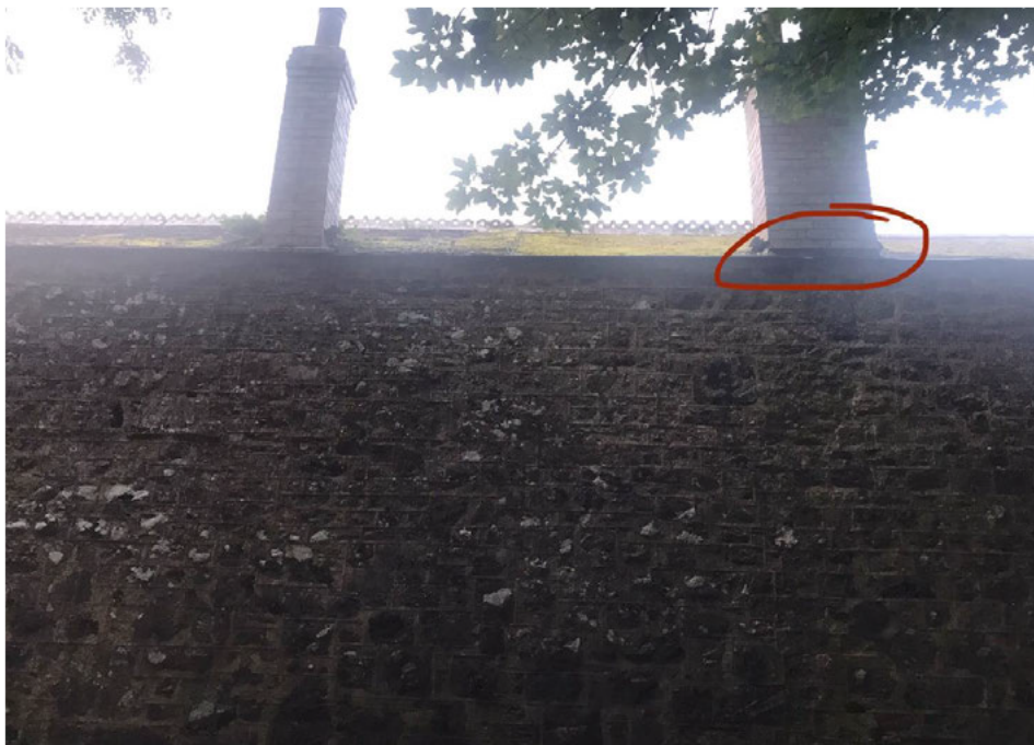
Figure 8: View of chimney on west elevation of cottages at Trereife House. Red circle shows approximate emergence location of common pipistrelle bat on 29 th August 2023 and 26 th September 2023.
