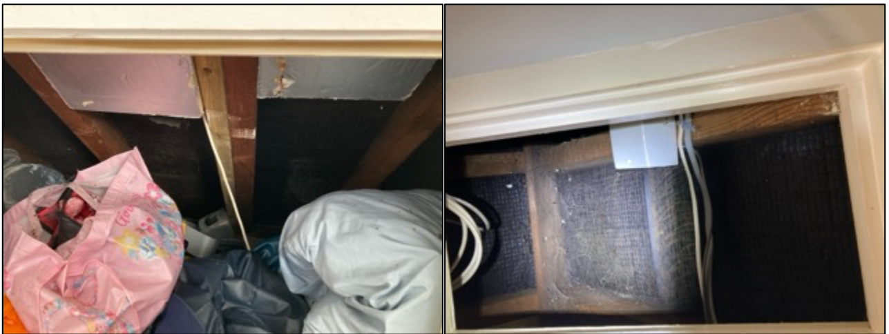
Photographs 2a (left) and 2b (right). 2a: Void 1. 2b: Void 2.
