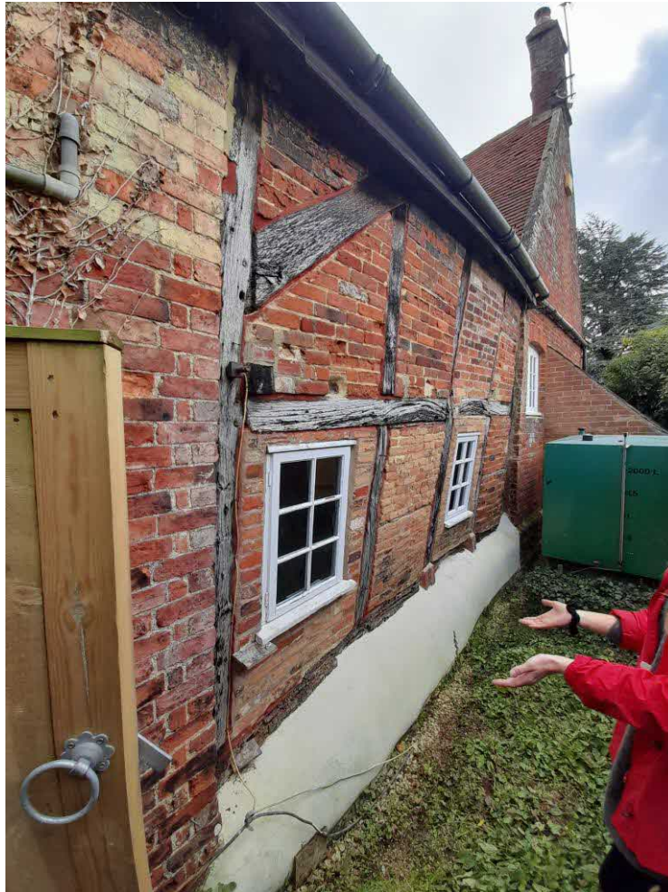
Photograph 15 Side angle of timber frame highlighting extensive bowing of wall
