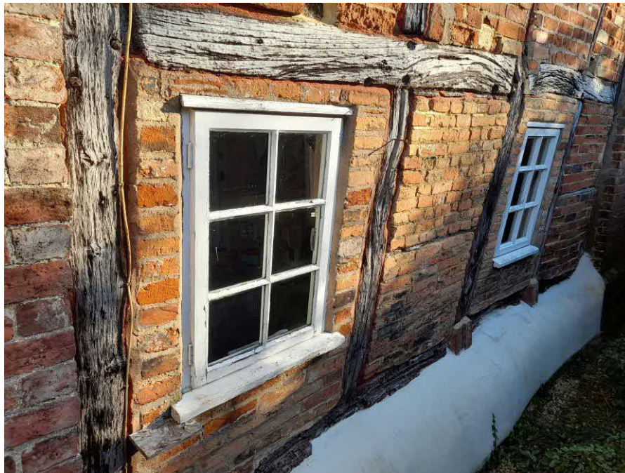
Photograph 3 Close up view showing poor condition of timber frame
