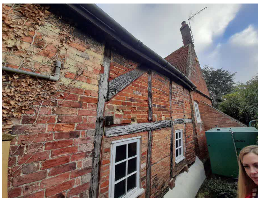
Photograph 2 North facing timber frame to original part of building requires extensive repairs
