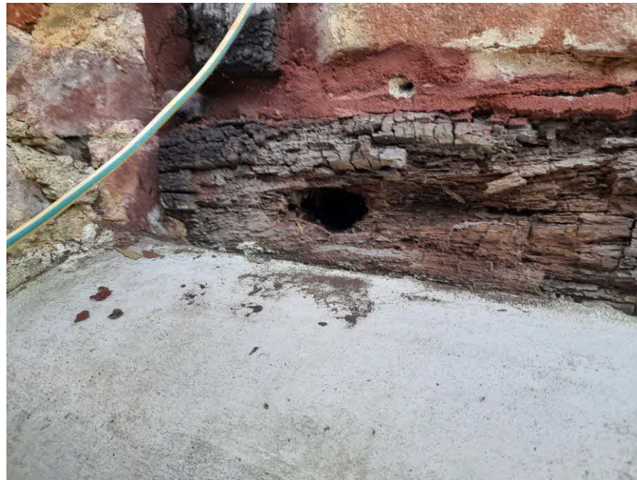
Photograph 16 Extensive decay & rat hole through sole plate to Playroom
