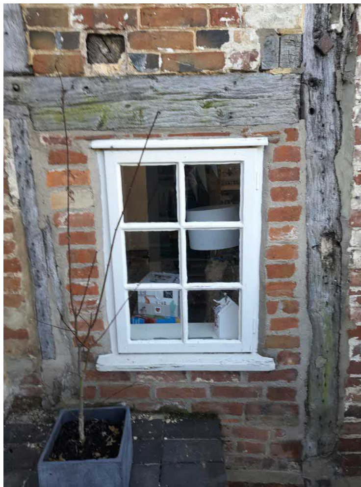
Photograph 9 Close up of modern window to be replaced, to right of porch
