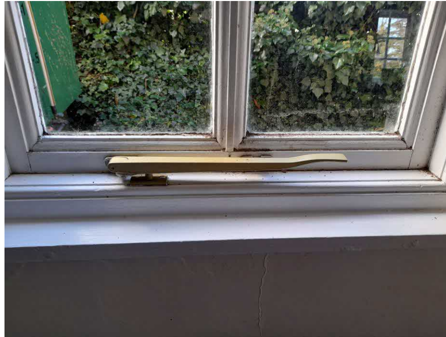
Photograph 18 Interior close up of window to be replaced showing thick glazing bars & modern inappropriate ironmongery
