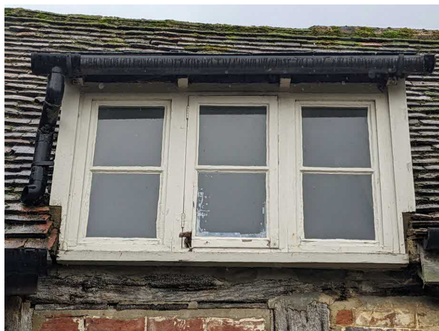
Photograph 14 External view of Bedroom window, showing poor condition of frame
