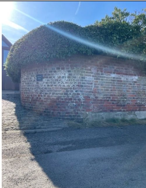
Image 1. View of the west end of the wall at the driveway return.
