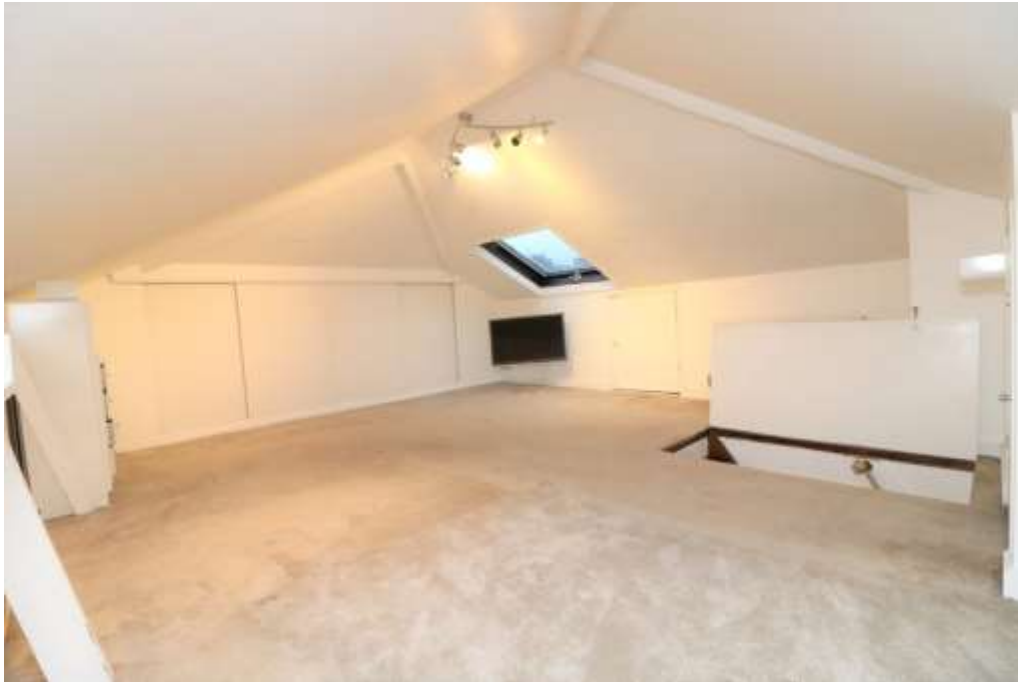
Figure 25 - View of the attic – with a single rooflight. Modern plasterboard to ceiling; low level plane timber panels closing-off the remaining roof area;
