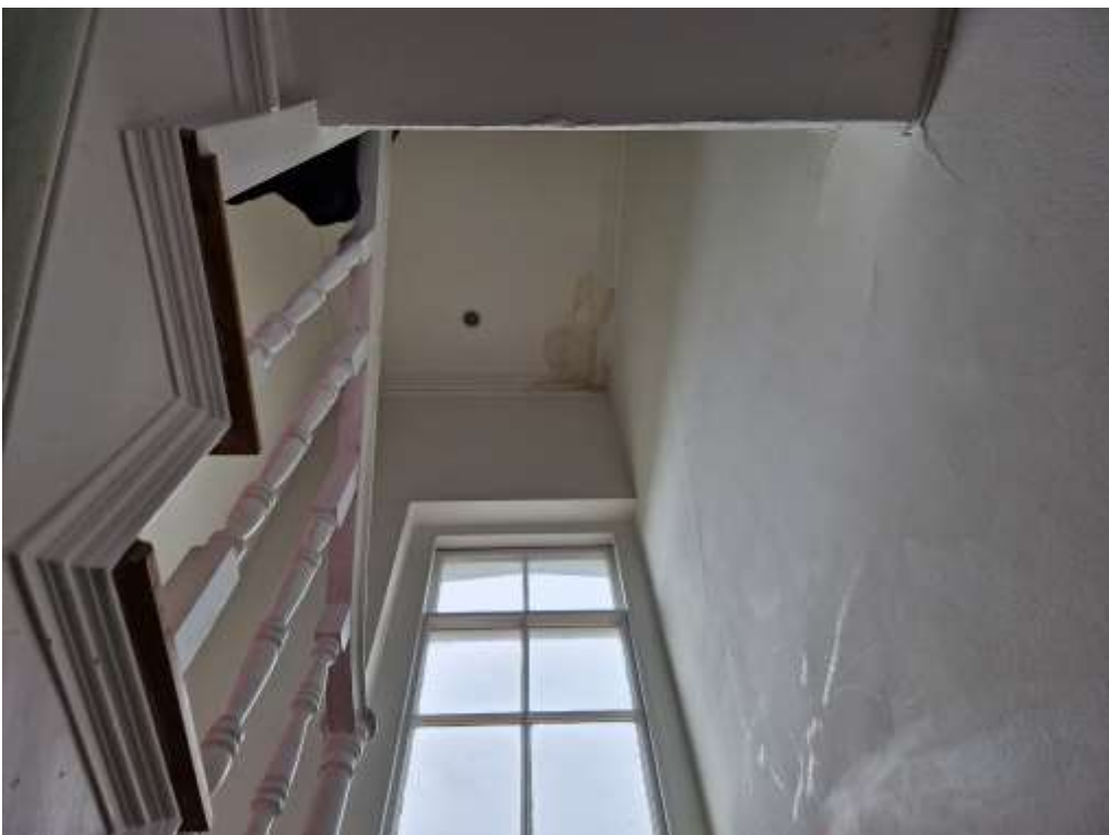
Figure 20 – stairwell, stairs, and the timber balustrade; ceiling damaged with the water ingress from the roof above;
