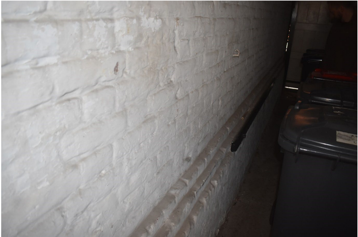
Figure 6. Previously external wall of 58 St Dunstan's Street, within the shared access passage.
