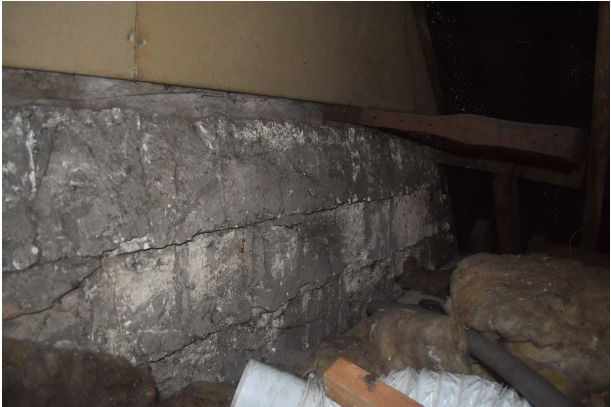
Figure 8. Formerly tiled external gable of 58 St Dunstan's Street within the roof space of No 59 (note bracket reinforcing connection of the two buildings).
