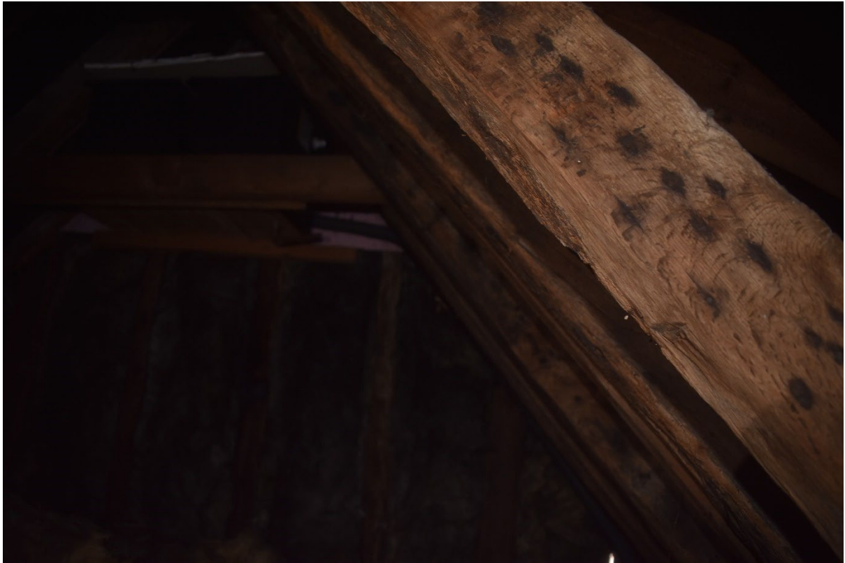
Figure 19. Nail marks in the reclaimed timber of the nineteenth-century roof within the later roof
