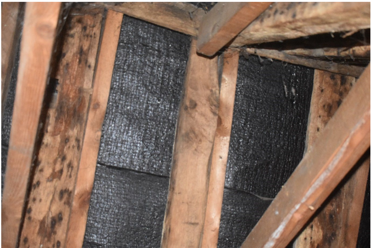
Figure 20. The somewhat distorted ridge board of the nineteenth-century roof
