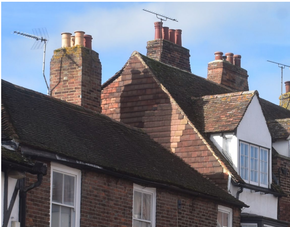
Figure 18. The same gable: external view. Note the change of pitch for the new roof to the left of the apex, and variations in tiles.
