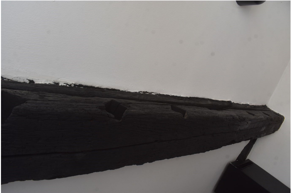
Figure 13. Reclaimed timber (with holes for mullions) in the timber frame on the first floor
