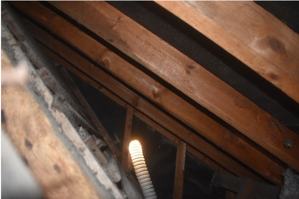
Figure 17. The nineteenth-century pitched roof with tile battens (left), within the later roof (right), looking towards south-west gable
