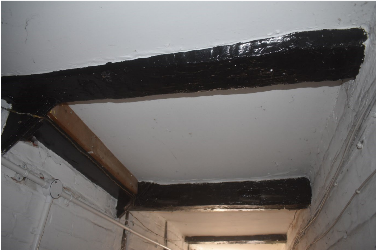
Figure 11. Reclaimed timber to form the first floor of 59 St Dunstan's Street (a former hatch at this location?).
