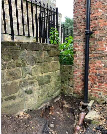
Figure 25 Drain to the south east of the Vicarage to be replaced
