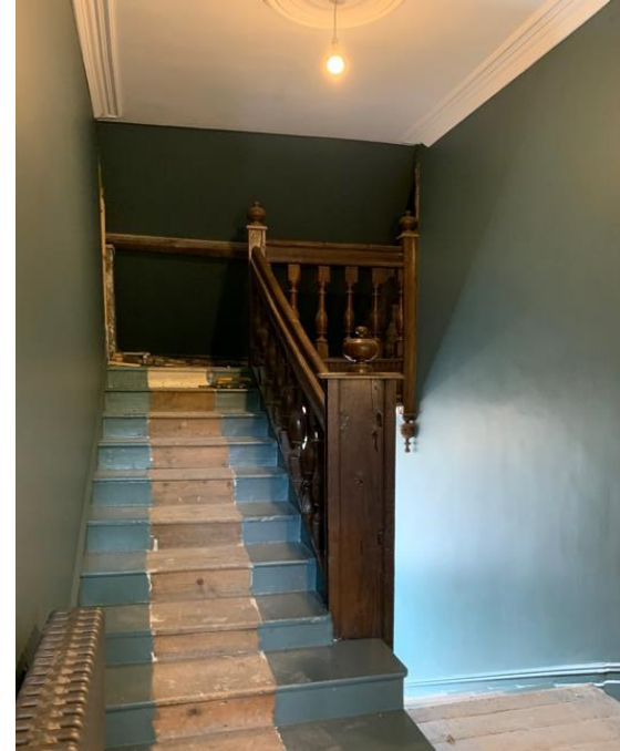
Figure 17. Area at second floor where a landing has been created to allow access into the loft through removal of modern partition.
