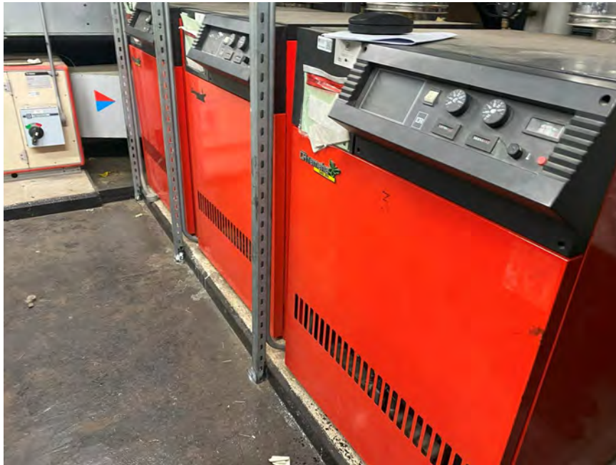
Fig 3: Block F Original Boiler Plant – Mezzanine Plantroom
