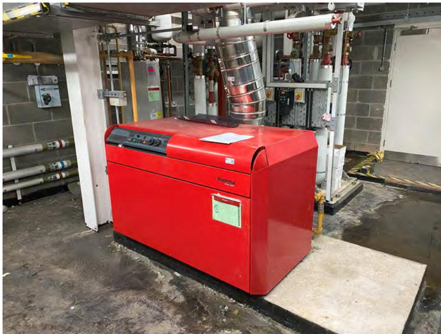
Fig 4: Block F Supplementary Boiler Plant – Third Floor Plantroom
