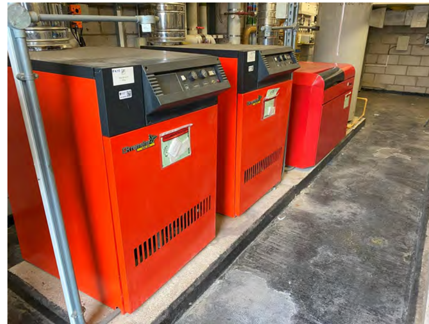
Fig 5: Block G Boiler Plant
