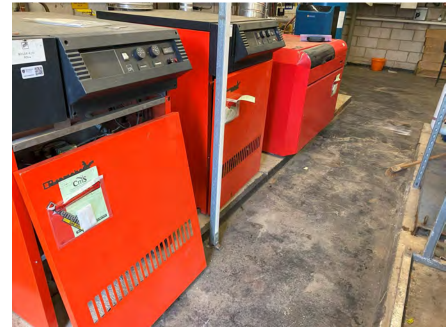
Fig 6: Block H Boiler Plant
