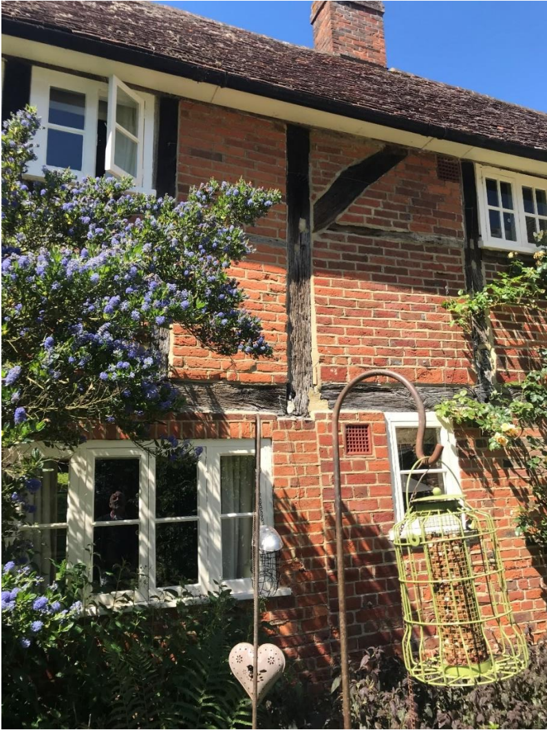
Figure 19: Detail showing the mixture of brickwork in the historic building.
