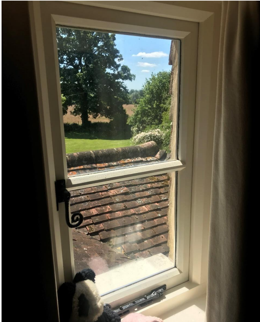
Figure 22: One of the modern windows in the south end wall of the first floor of the historic building. View over the 2000 extension roof.
