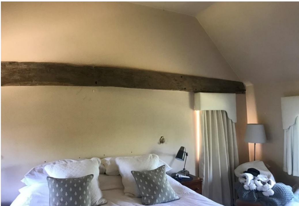
Figure 21: Interior of the first-floor south room of the historic building, looking towards the south end wall which would connect through to the proposed extension. There are modern windows either side of the south end wall.
