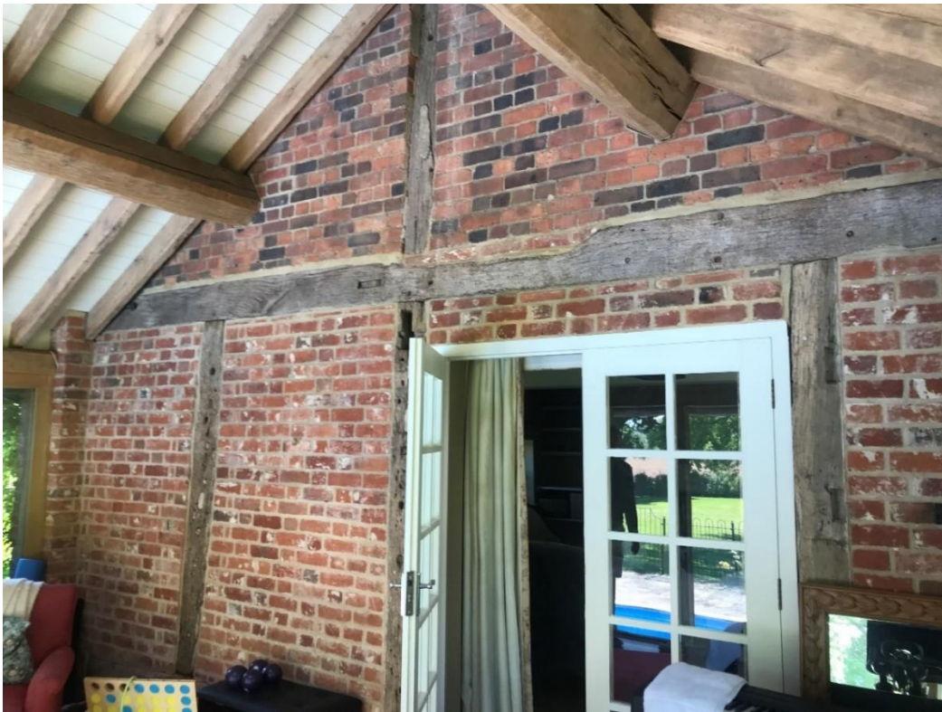
Figure 20: Interior of the 2000 conservatory extension, looking toward the south wall of the historic building.
