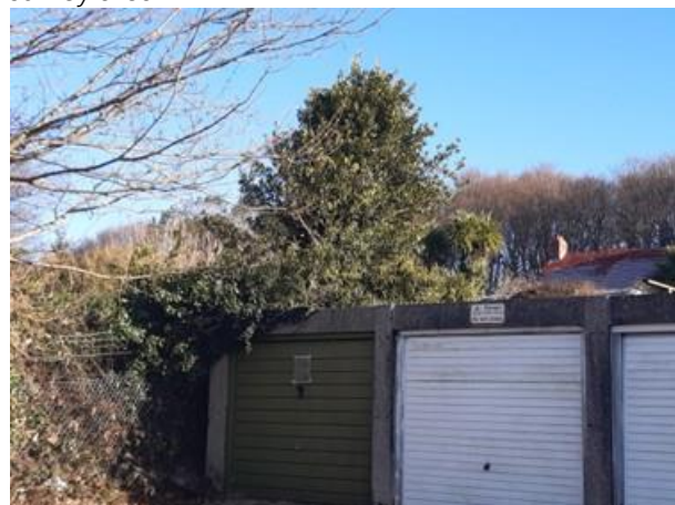
TN8 Dense ivy on northernmost garage roof in the south-east of the survey area.
