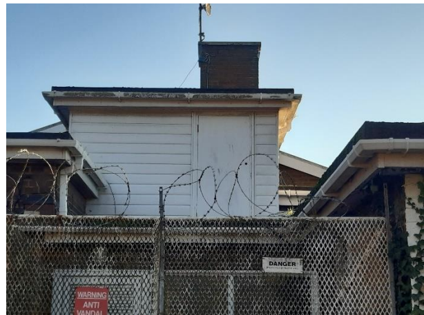
Small water storage room on the roof of the building which was not accessed during this survey.
