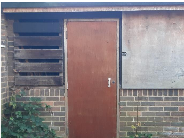
Northern extension with large gaps between planks allowing potential access by bats to the interior of this room.
