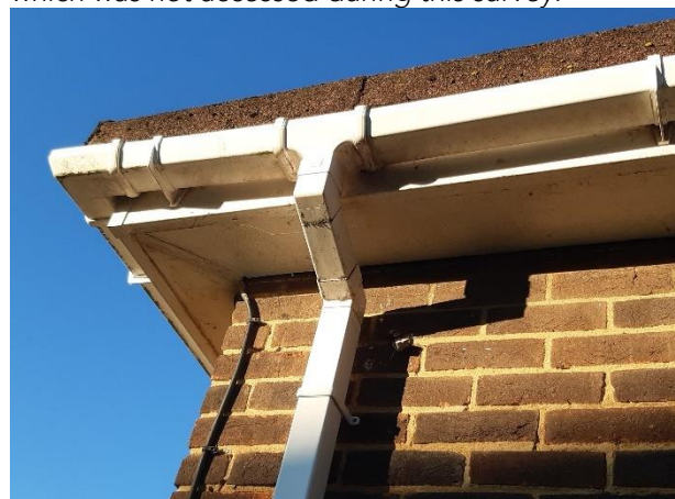
The gutters, soffits and fascias of the building are in a reasonable condition.
