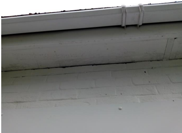
Gaps in fascia to northern aspect
