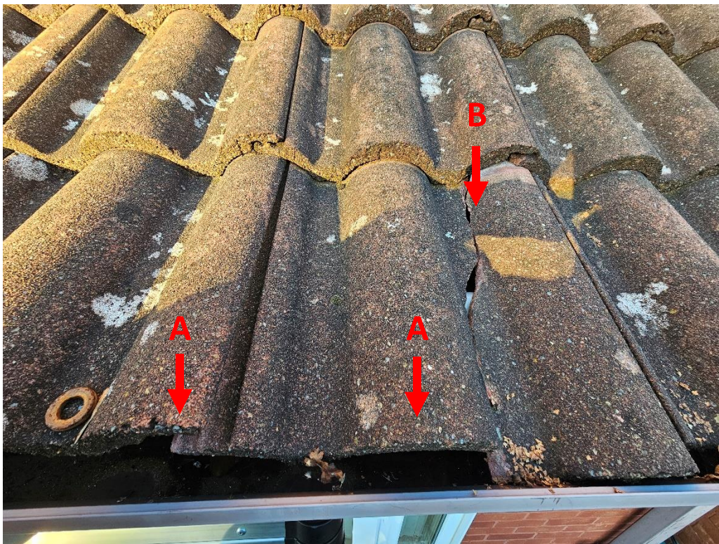
Plate 6. Raised tiles (A) and broken tile (B) on the pent-roof section.
